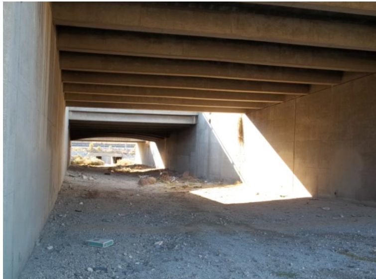
Figure 4. Photograph of a characteristic atrium taken from the entrance of Stubbe West underpass. The atrium is an opening in the underpass where the two directions of highway traffic are separated allowing for light to naturally illuminate the underpass.
