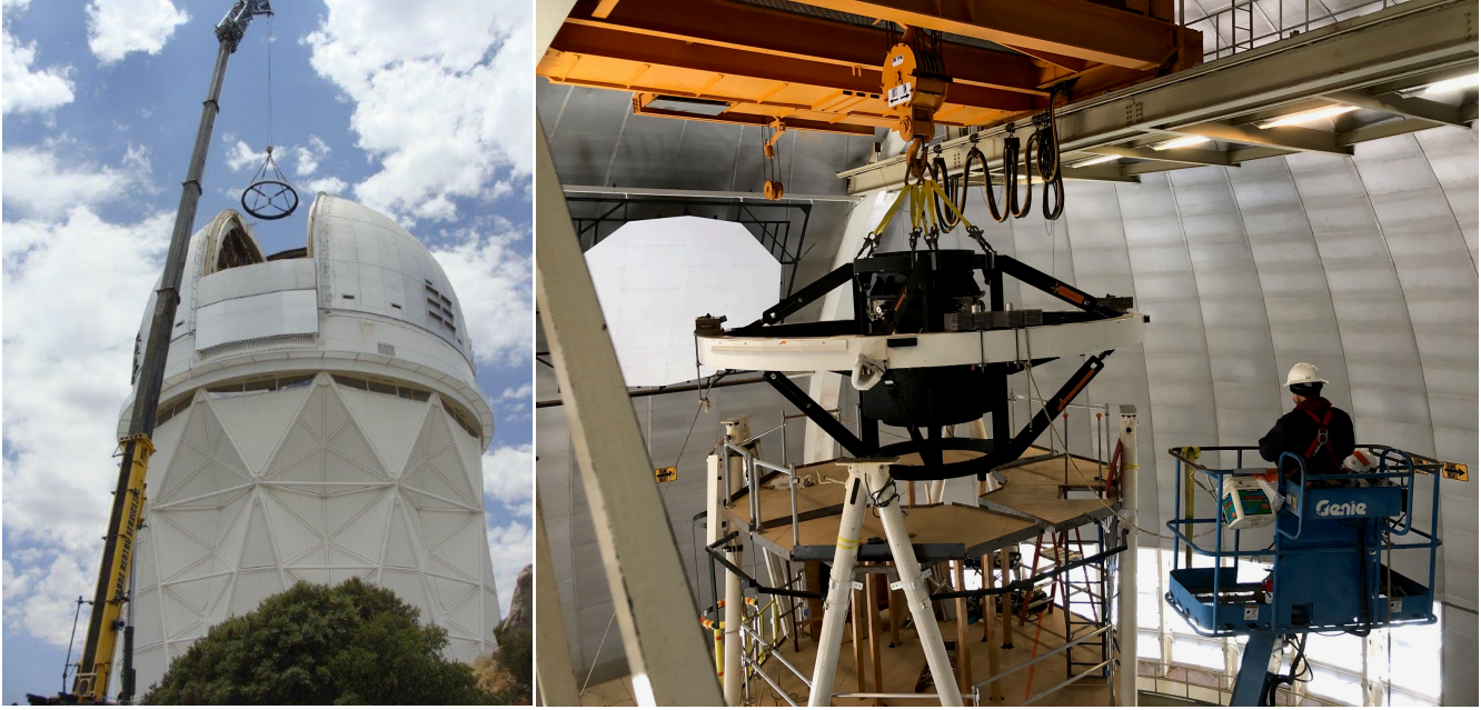
Figure 23. Installation phases of the new top ring. ( Left ) Transfer of the new top ring from the ground level to the dome floor via the dome slit with a 450 ton crane on 14 June 2018. The same crane was used to remove the old top end. ( Right ) Installation of the fully assembled, new top end with cage, hexapod, and corrector barrel to the Mayall’s Serrurier truss on 28 November 2018.
