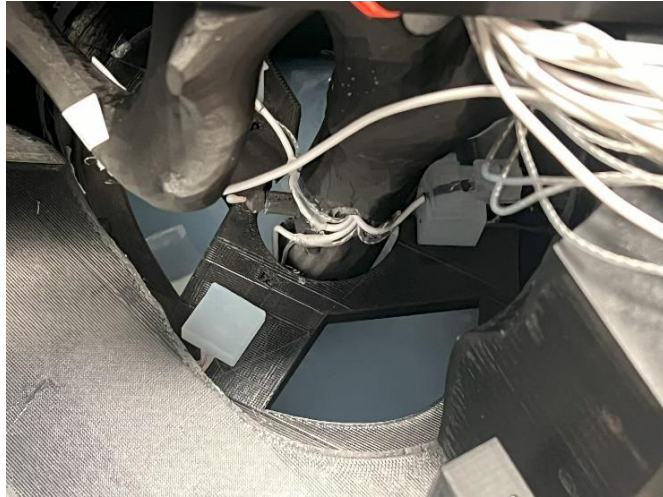
Figure 68: The removable template used to position sensors at the correct level, prepared for the 4th pour.
