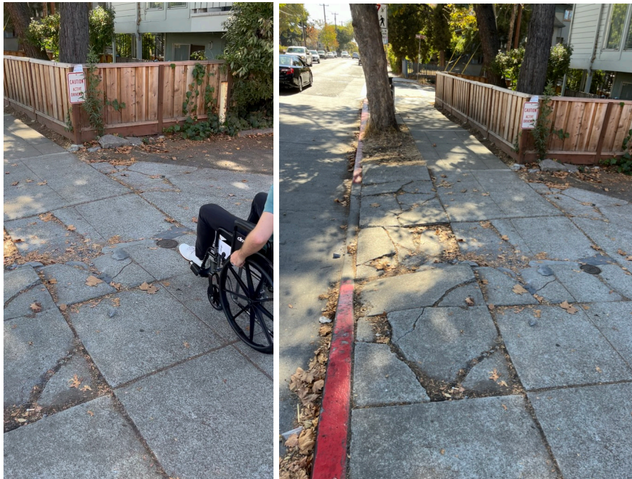
Figure 4.17: Uneven sidewalk and tripping hazards
