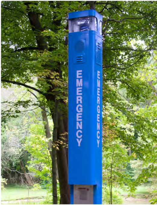
Figure 76: Emergency phone in park.
