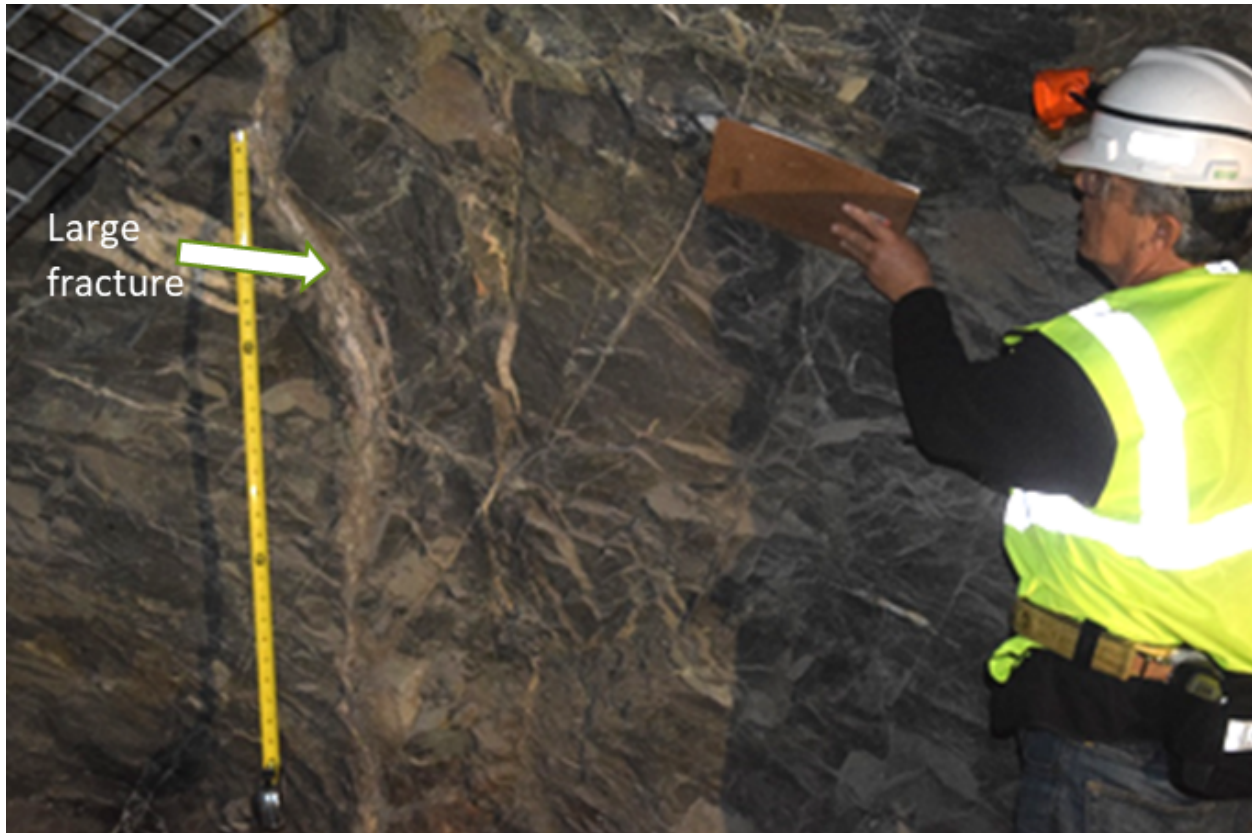
Figure 3. Large fracture near the tape measure for scale (intervals on the tape are 1 ft). The fracture is filled in this photograph but other, similar fractures are exposed in the drift with open space.
