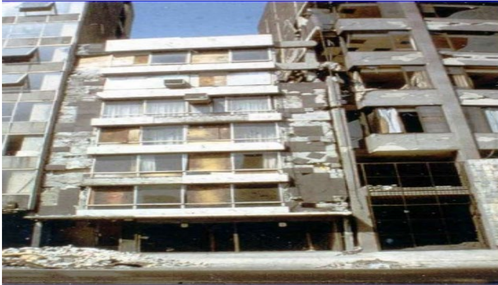
Figure 2.2. Pounding-induced damage in adjacent buildings following the 1985 Mexico City earthquake. Photo credit: Walter Hays, Global Institute for Energy and Environmental Systems.
