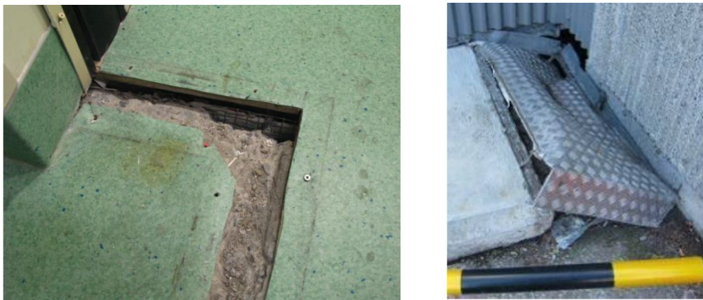
Figure 2.20. Damage to a seismic gap cover as a result of moat wall pounding during the 2010 Darfield earthquake [61].
