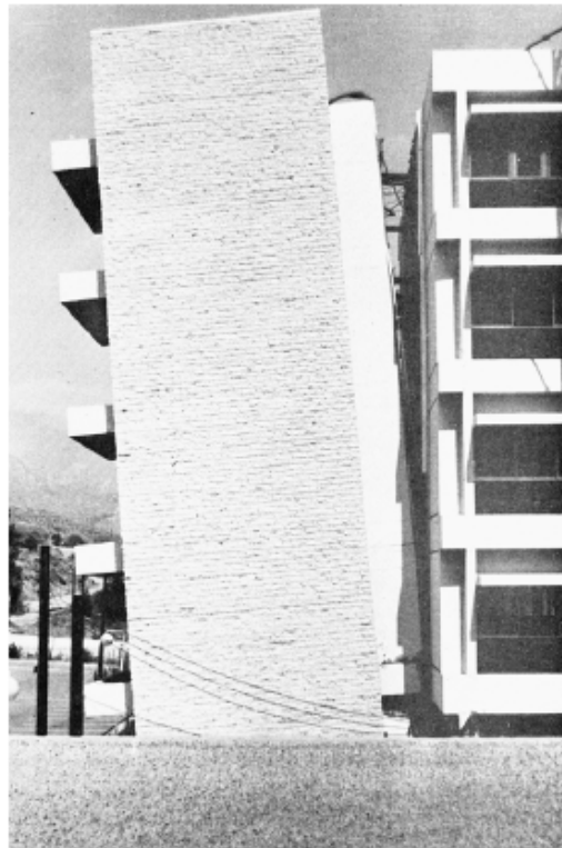
Figure 2.1. Permanent tilting in a stairway tower caused by seismic pounding in the 1971 San Fernando earthquake [1].
