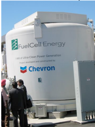
Fig. 2. The 1 MW Fuel Cell at Santa Rita Jail
