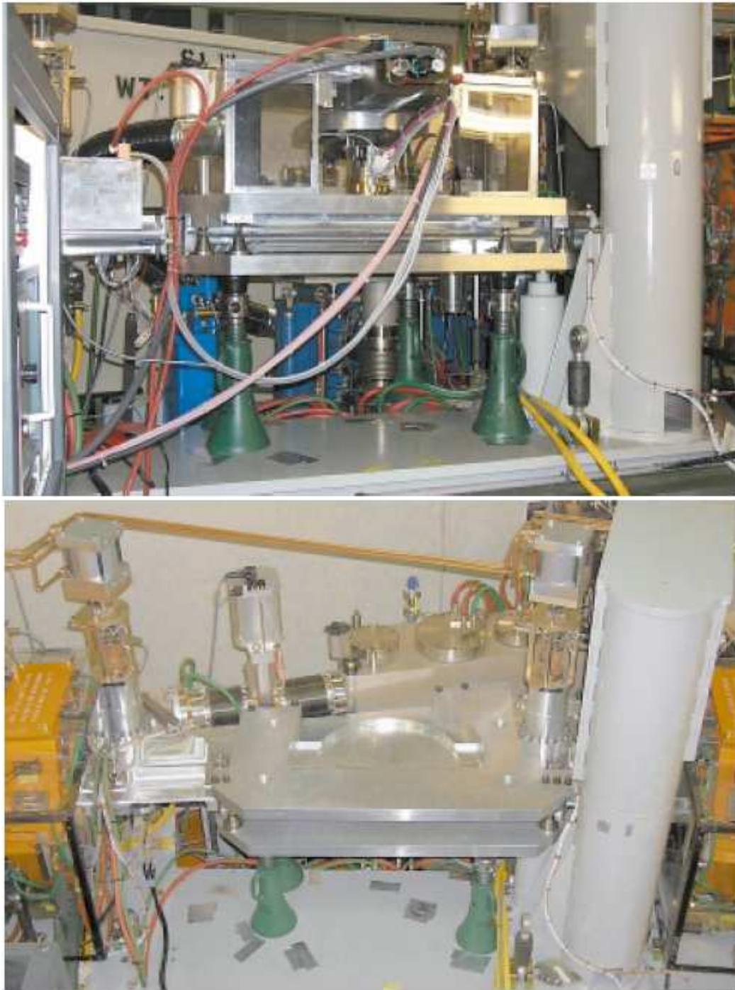
Fig. 14. The left photograph shows fixtures and tools used to machine the ALS aluminum vacuum chambers in situ, in preparation for the Superbend installation. The right photo shows the finished circular cut out for the Superbend cryostat.
