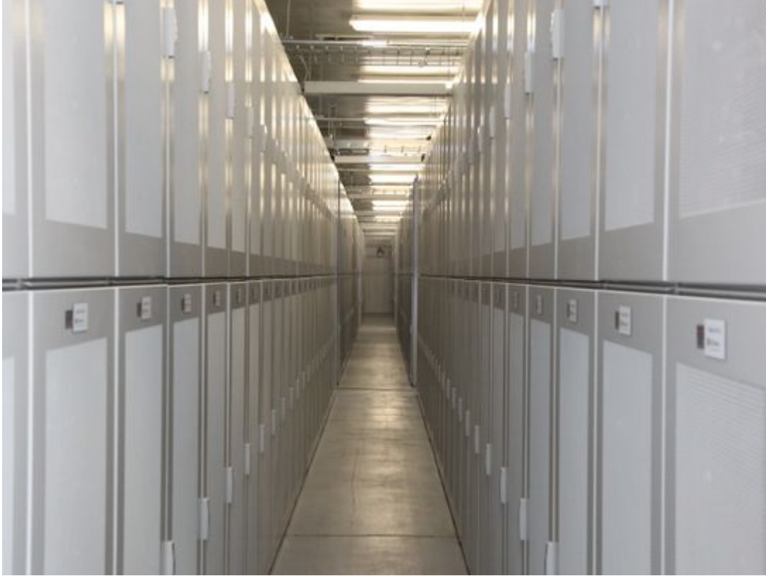
Figure 22. A 32-megawatt-hour lithium-ion energy storage project at the Monolith substation in the Tehachapi Mountains of California, USA
