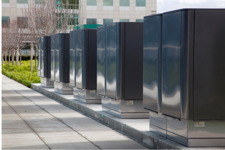
Figure 20. Bloom Energy fuel-cell power system
