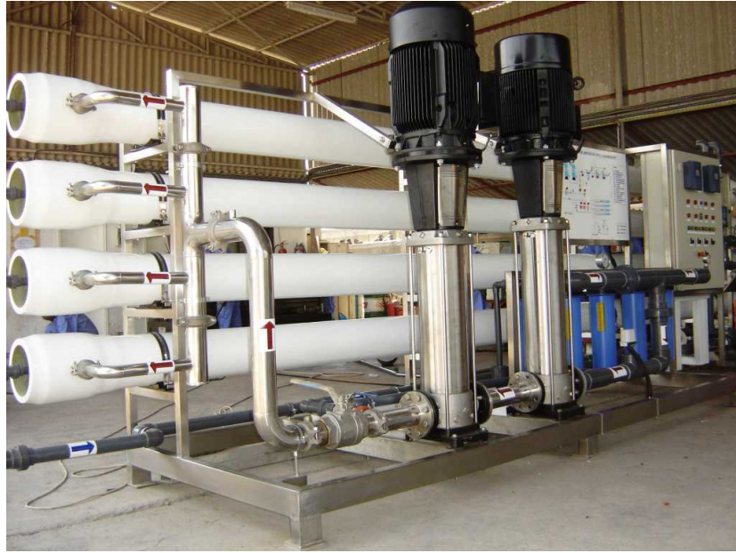
Figure 36. Reverse osmosis equipment at an industrial facility
