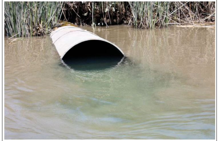
An outflow pipe from the City of Fairfield Municipal Wastewater Treatment Facility in Boynton Slough. Although this effluent has undergone tertiary treatment, it still contains low concentrations of endocrine disrupting compounds. Credit: S. Brander
