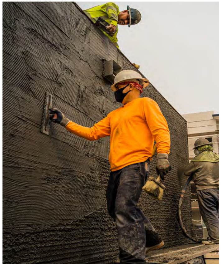
Construction of Vista Verde Apartments in Ontario during the COVID-19 pandemic. Photo credit: City of Ontario
