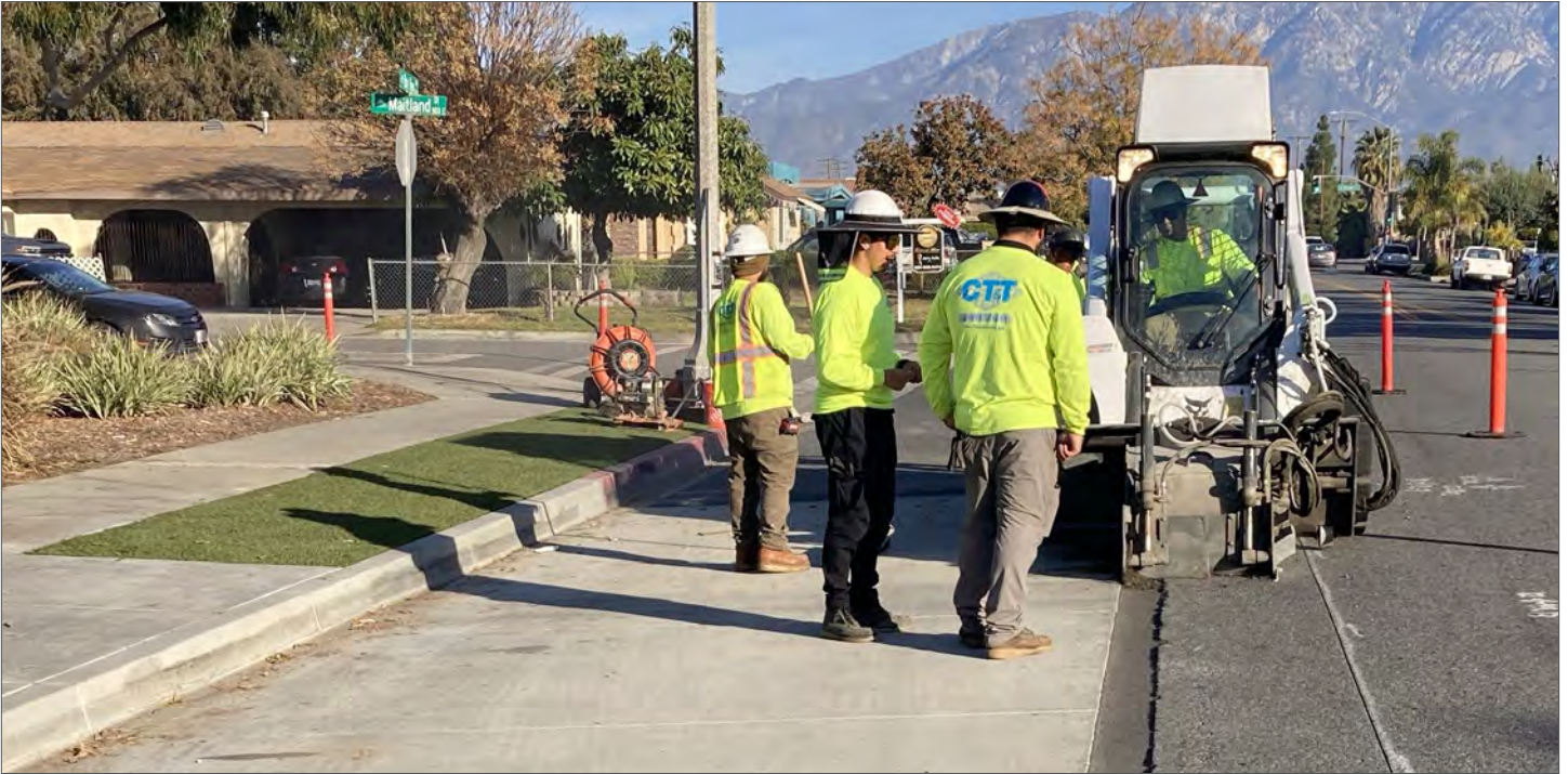
Crew works on construction of missing sidewalk segment, including bus pad installation, for the Pedestrian Pathway Improvement and Network Connectivity Project. Photo credit: City of Ontario
