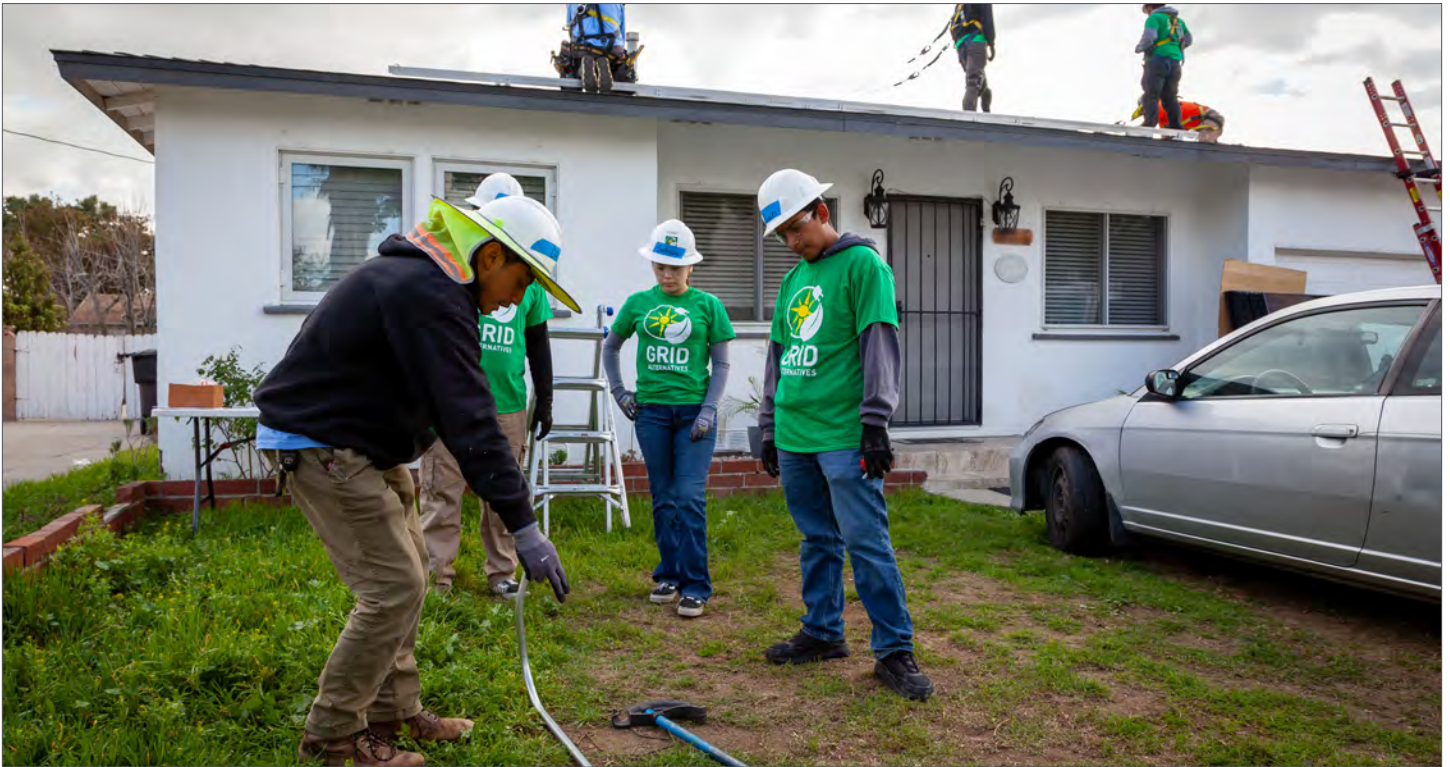
GRID Alternatives staff and high school students install solar panels on a single-family home. Photo credit: GRID Alternatives
