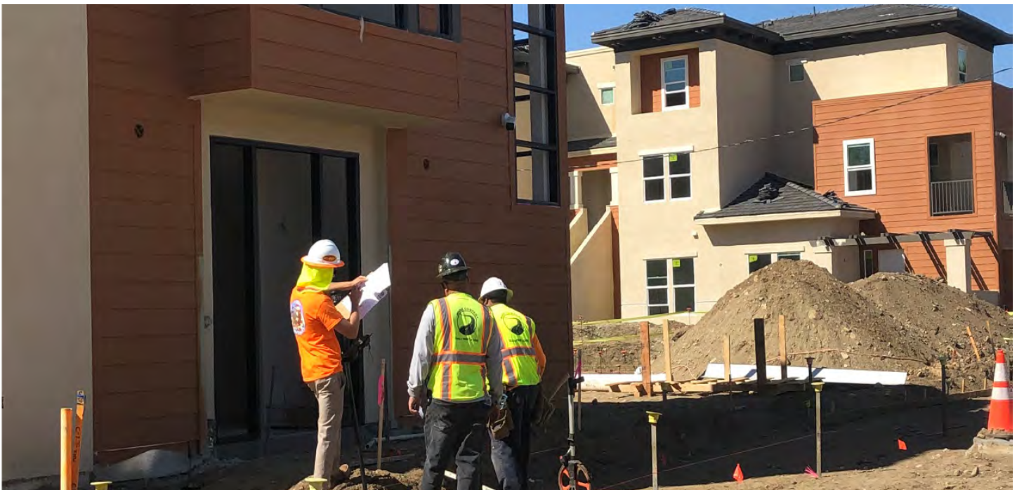
Construction of Emporia Place Apartments in Ontario, a Displacement Avoidance Plan project. Photo credit: City of Ontario
