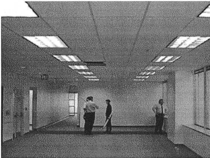
Figure 2. An interior view of the third floor taken during commissioning of the lighting system before installation of the furniture system. Note the luminance pattern on the far wall which shows that the row of lights nearest the window is heavily dimmed while the second row is at near full intensity.
