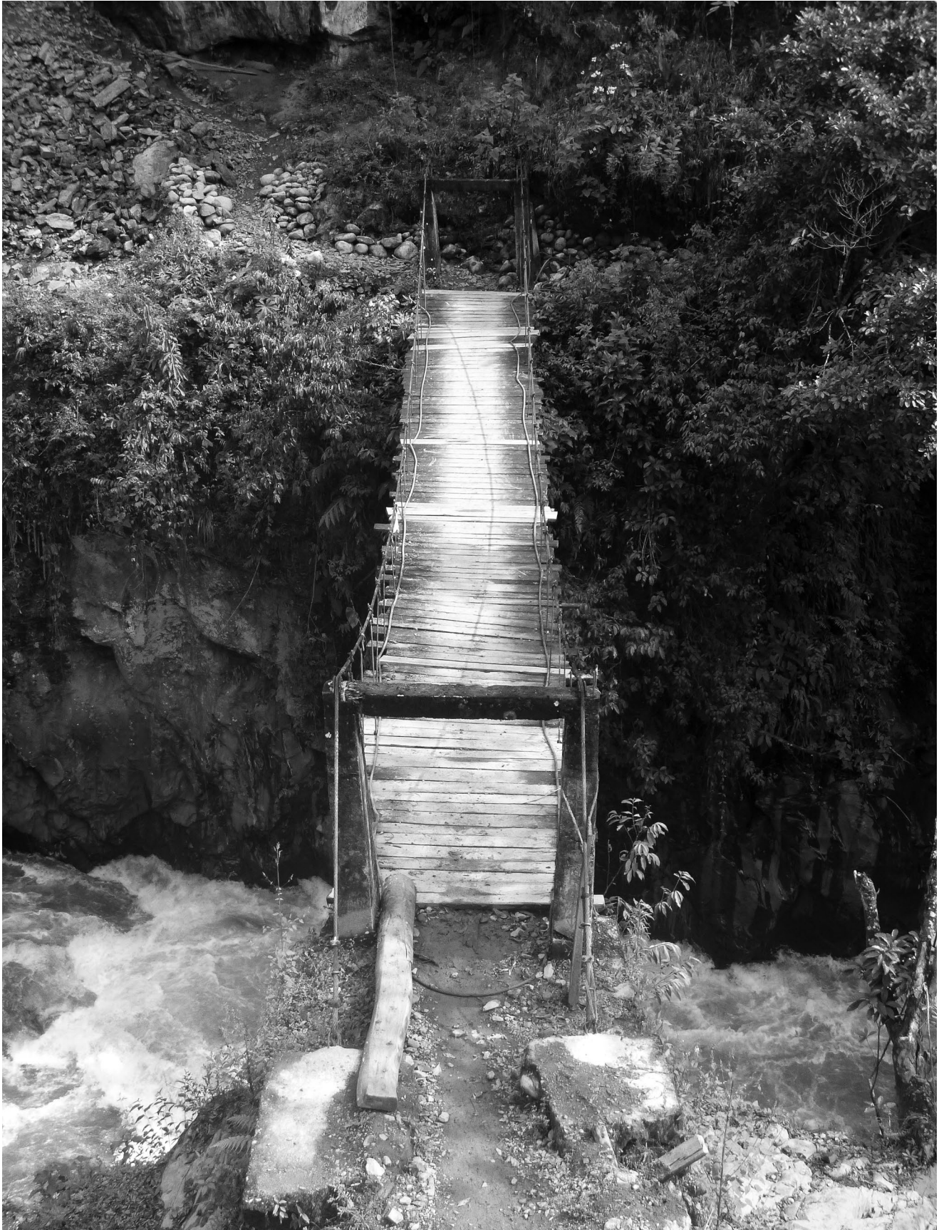
Figure P.2. The Azulmayo Bridge, 2010 (photograph by Brian S. Bauer and Miriam Aráoz Silva).
