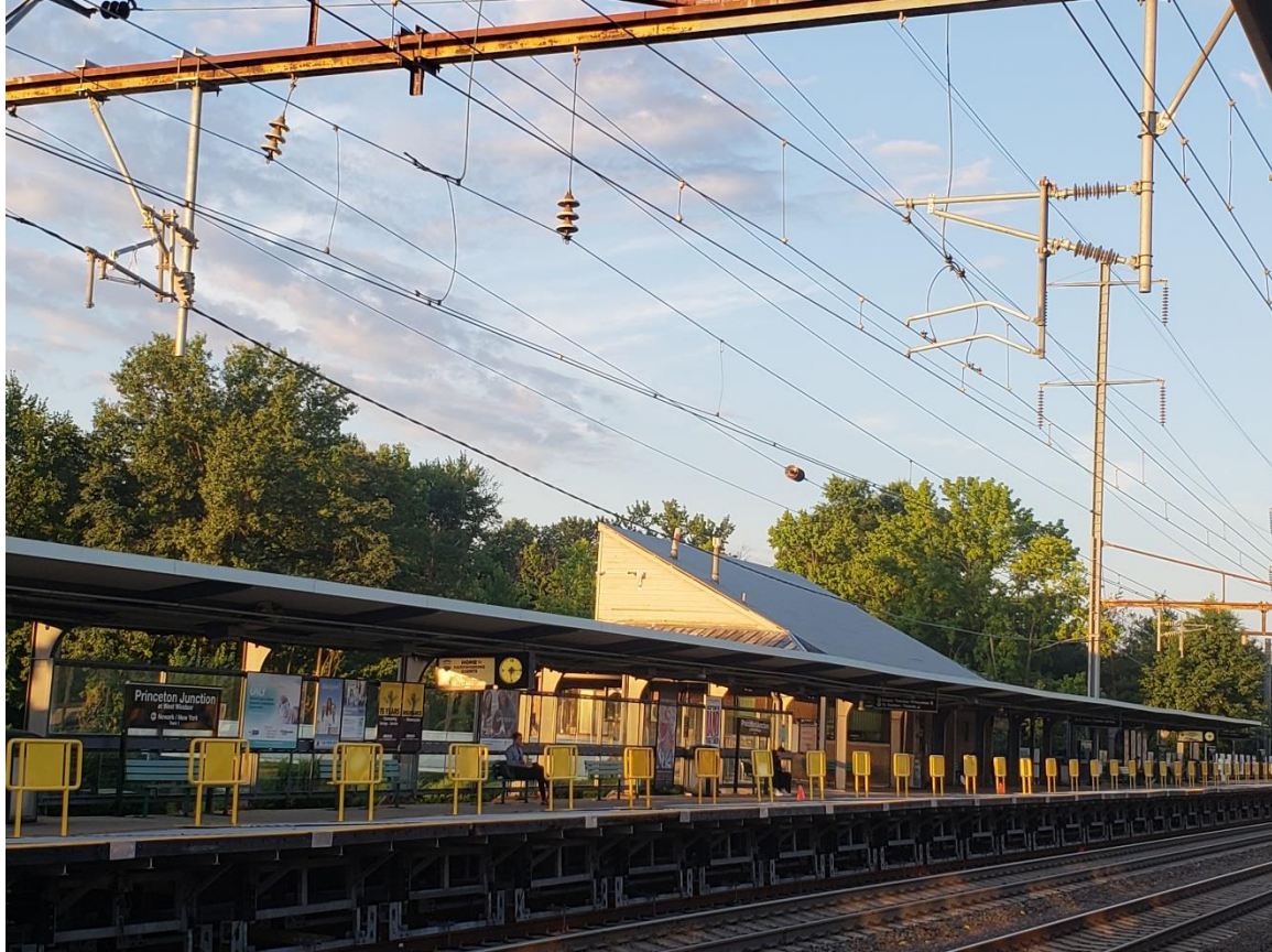
Figure 3: OLE Infrastructure at the Princeton Junction Train Station, Princeton, NJ
