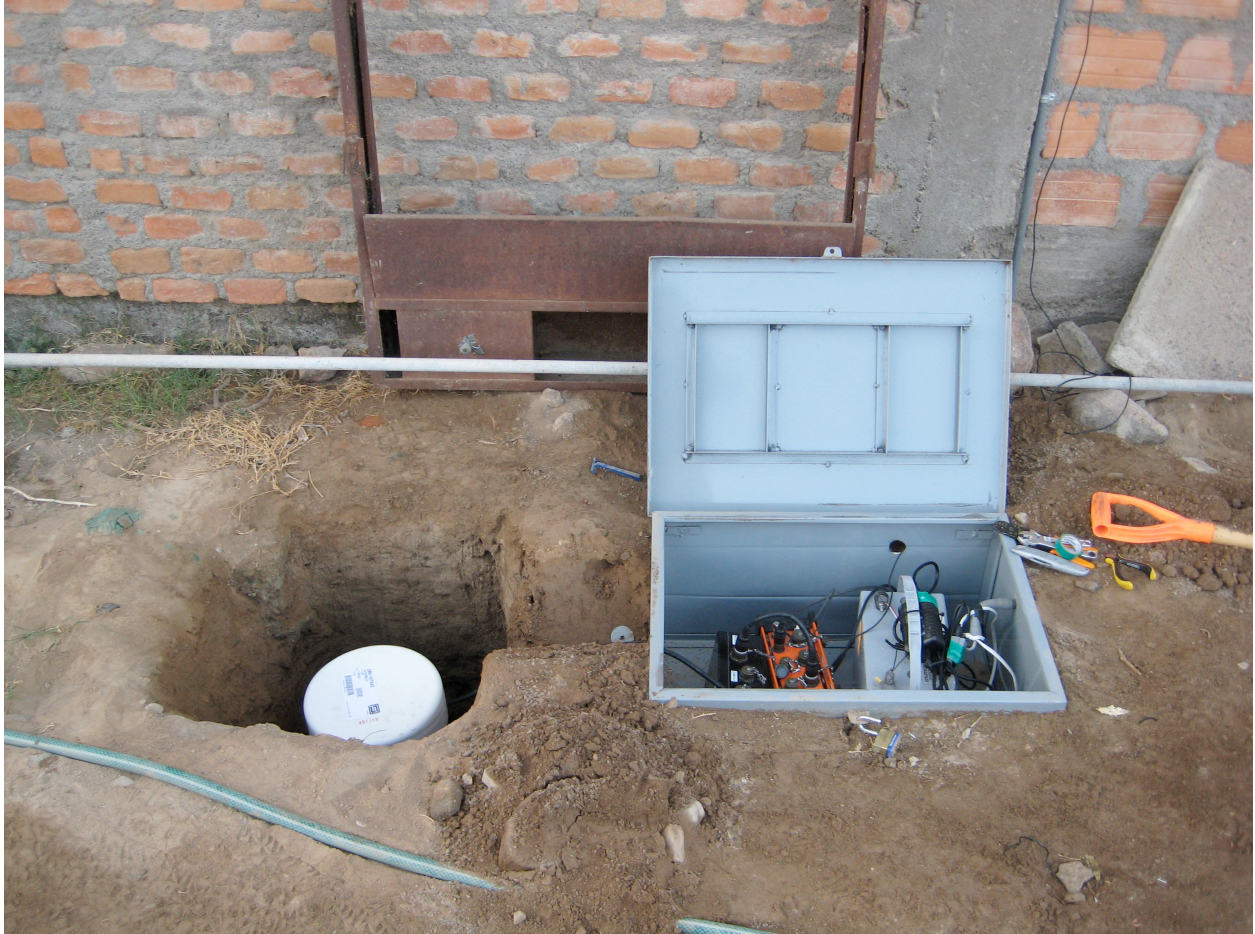
Figure 1 – Seismic sensor installation in Peru (photo taken in 2008)
