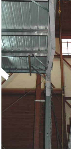
(a) South Rafter Lateral Buckling
