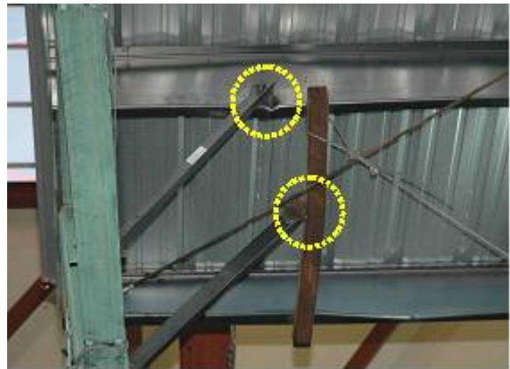
(b) Overload of Brace Support
