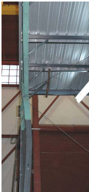
(a) South Column Lateral Buckling
