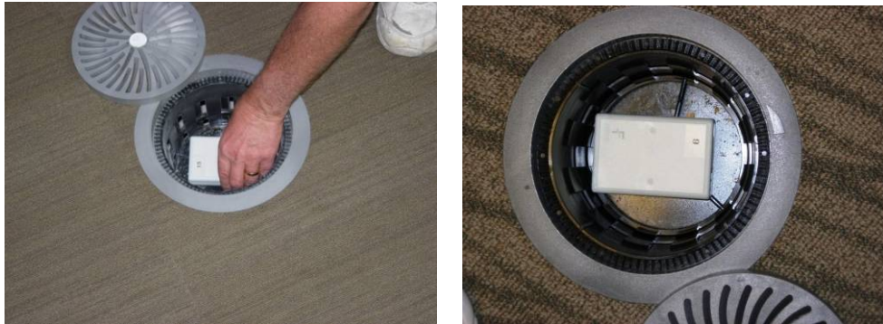
Figure 12: Mote placement in diffusers
