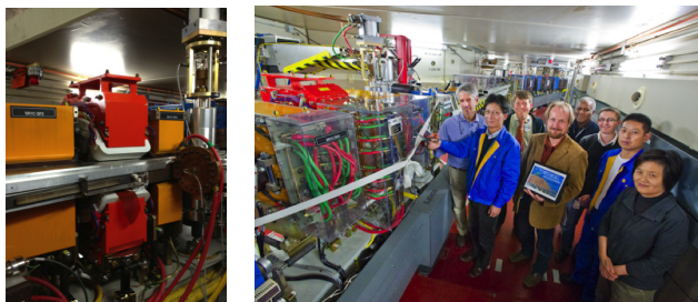
Figure 5: Left: SHD magnet installed between the QF and QD quadrupoles. Right: Ribbon capping celebration after successful installation.
