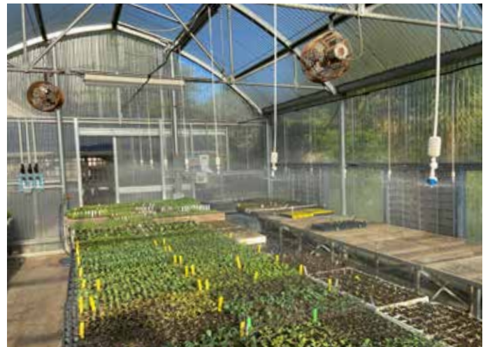
FIGURE 23. Typical 3/4" solenoid valves with screen filters to prevent debris from clogging sprinkler nozzles. Three bench, three valve layout, controller in right rear of photo, valves for each station in left rear of photo and sprinkler nozzles arrayed evenly over each bench to provide uniform water delivery. Photos: Christof Bernau
