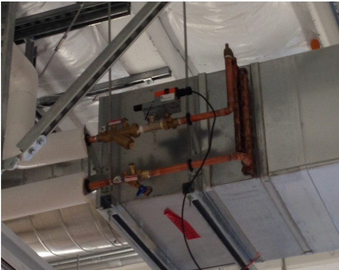
Figure 8 – Typical hot water pipe installation at VAV reheat coil with uninsulated piping and fittings.
