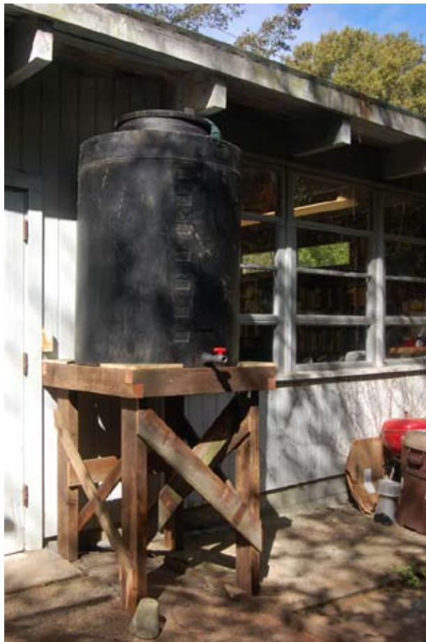
A cistern catches rainwater from the roof which is then used to irrigate the surrounding landscape plantings.
