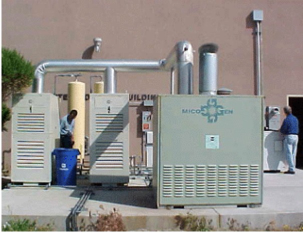
Figure 10. Installation at the Santa Margarita Water District digester plant.
