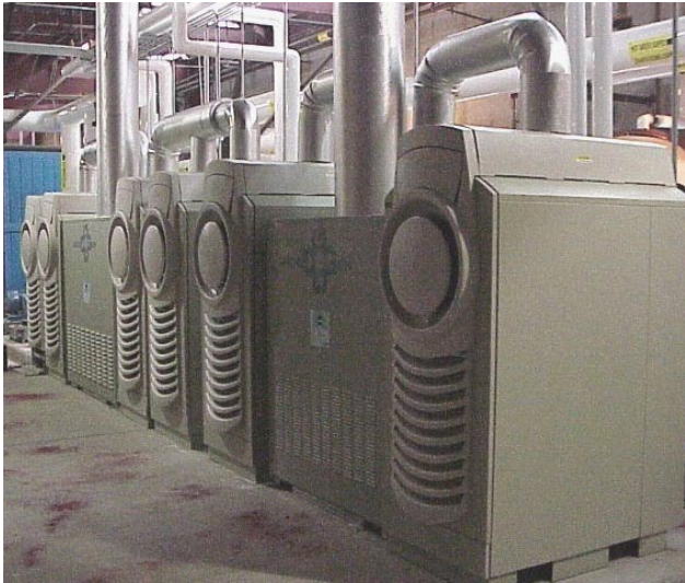
Figure 9. Installation at CSUN Central Plant.
