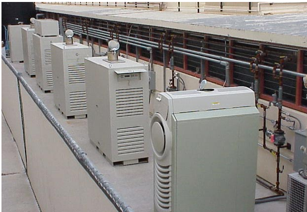
Figure 12. Installation at UC Irvine.
