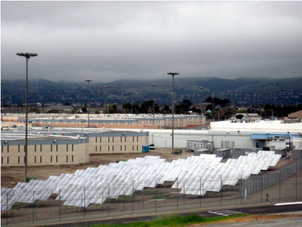
Figure 17: Recent photo of Santa Rita jail with ground mounted tracking solar PV in foreground and batteries and fuel cell directly behind
