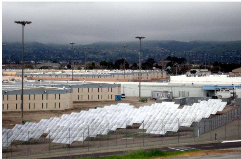
Figure 3: Recent photo of Santa Rita jail with ground mounted tracking solar PV in foreground and batteries and fuel cell directly behind
