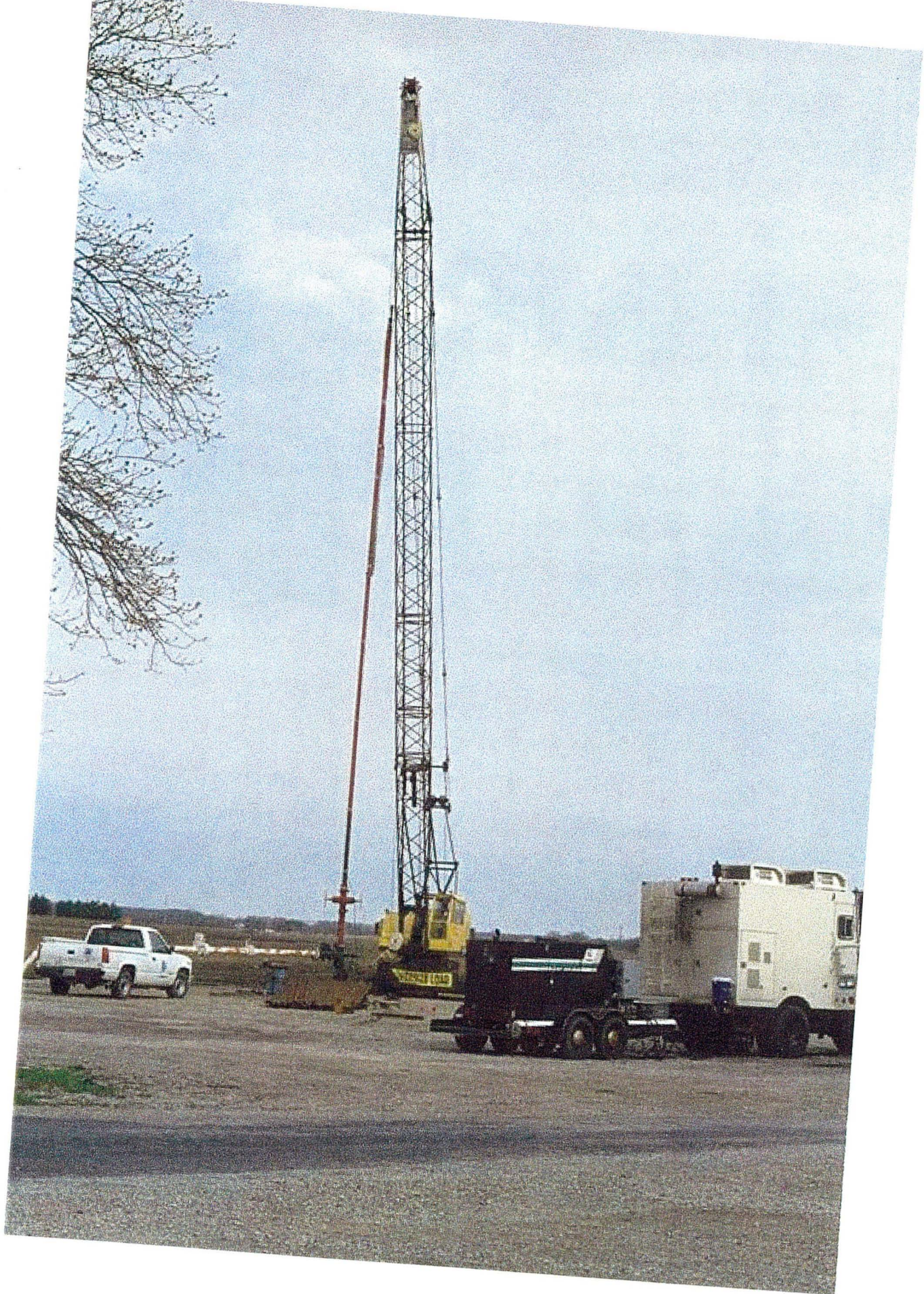
Figure 5. Sixty ft. lubricator pipe used to introduce multi-level sensor string in the pressurized VSP well.
