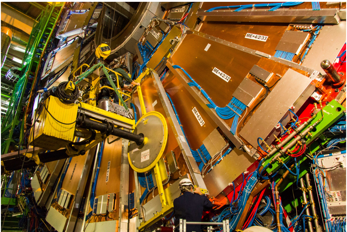
Figure F.3: A closeup of the crane fixture used to install CSCs in the CMS Cavern.
