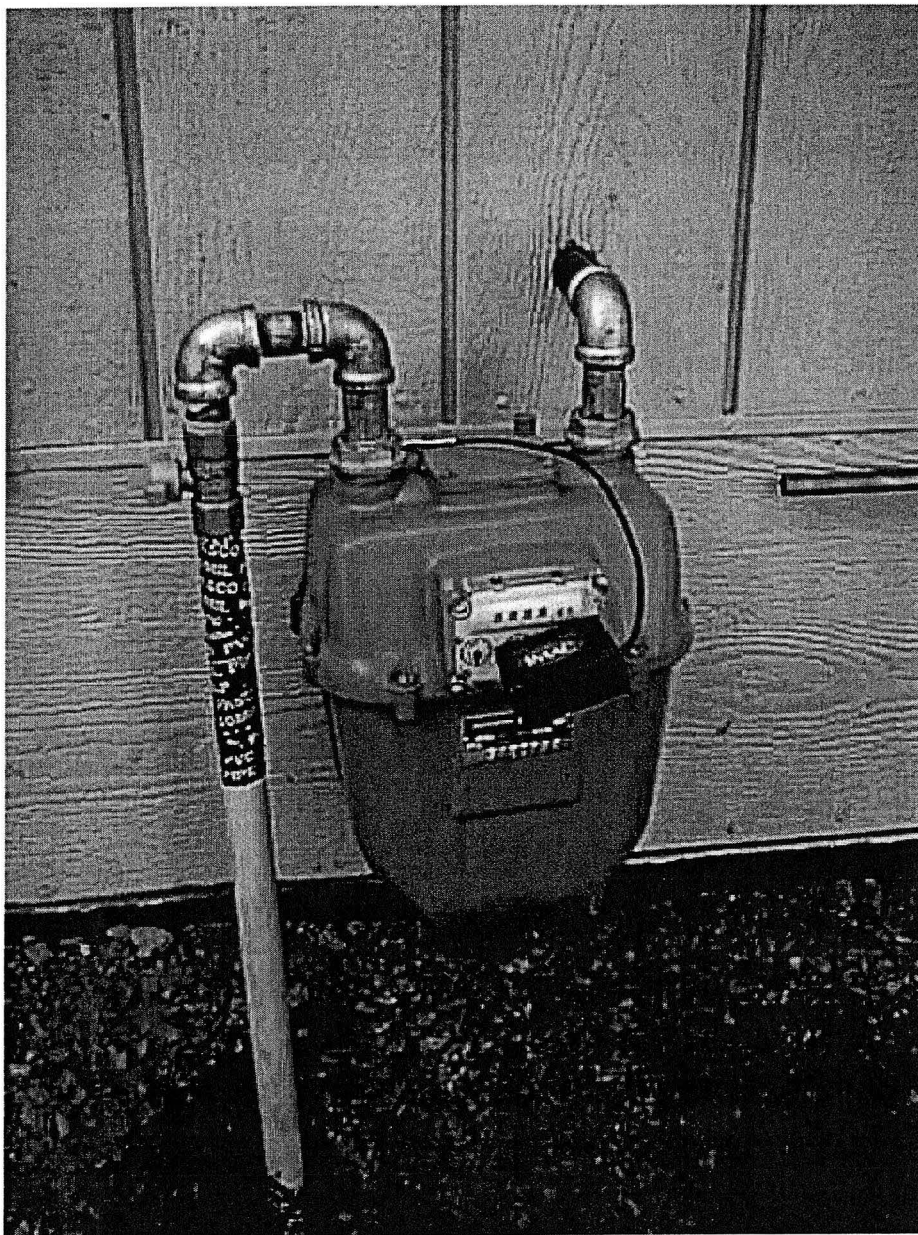
Figure 11: Photograph of the advanced HVAC system's water heater gas usage sensor (Equimeter 275P) for the energy monitoring component of the field study.
