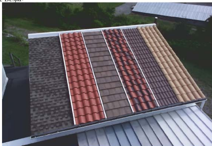
Figure 4. Testing cool-colored roof materials at Oak Ridge National Laboratory on the Envelope Systems Research Apparatus.
