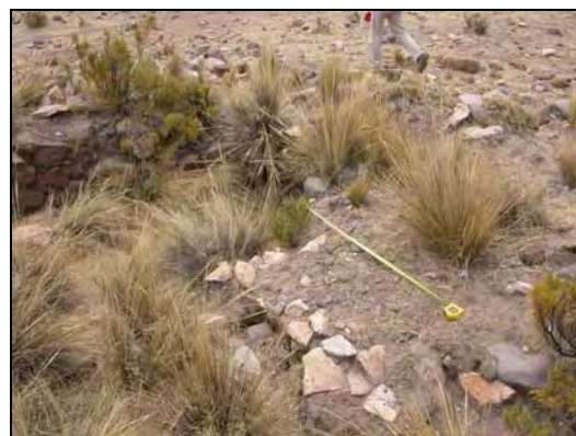
Figure 6-84. Collapsed wall of A03-663 structure.
