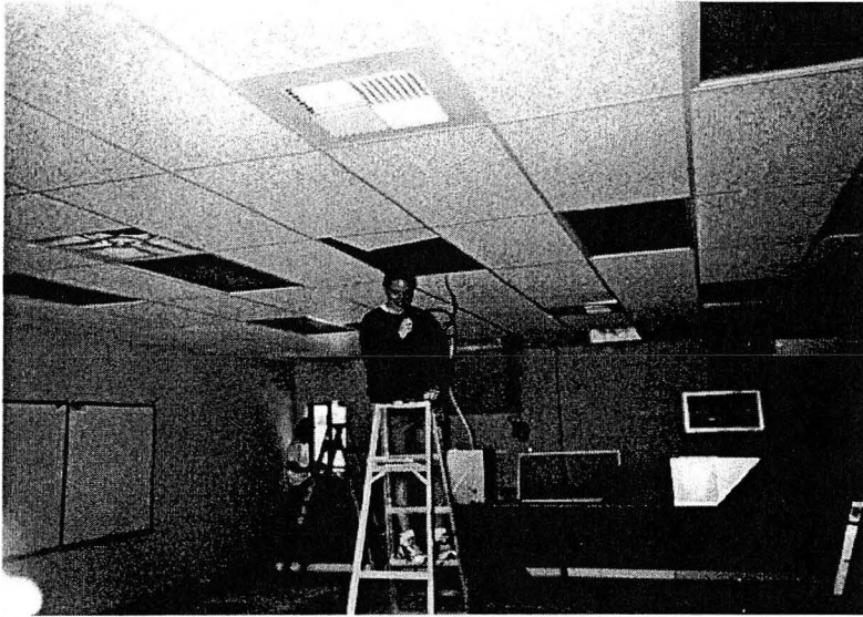
Figure 17 (a-c): Photographs of LBNL designed Lexan mobile located at the center of each RC 1-2 ft down from ceiling, i.e., 6.5 ft above carpeted floor, for SLM (noise level, dB (A)), T and RH measurements, including (a) installation, (b) SLM calibration and (c) co-located Quest M-27 noise dosimeters to validate the orientation and location of the SLM microphone.
