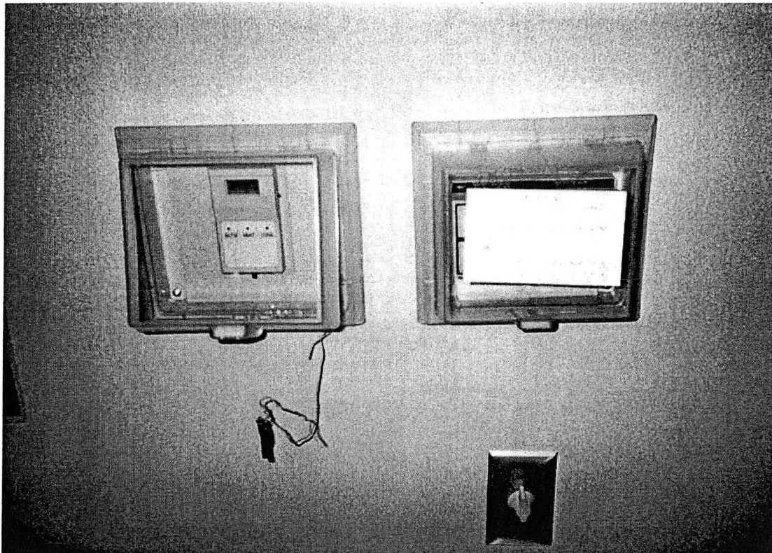
Figure 5: Side-by-side control thermostats for IDEC and standard HVAC systems in each field study RC. Plastic lock boxes and notes were used to remind teachers which system to use during the school year, given the case-crossover study design.
