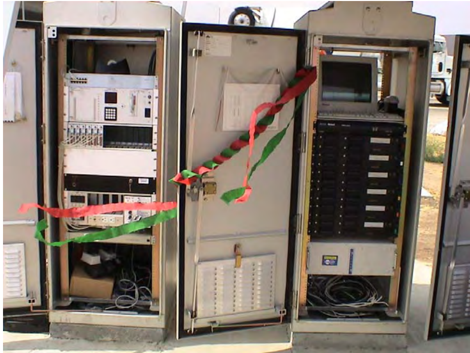
Figure 5.2 Field traffic cabinets
