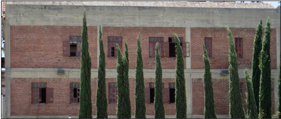
Figure 105: The back of the Annex faces the hotel's employee parking lot. The windows are left open or broken out. Photo by author.
