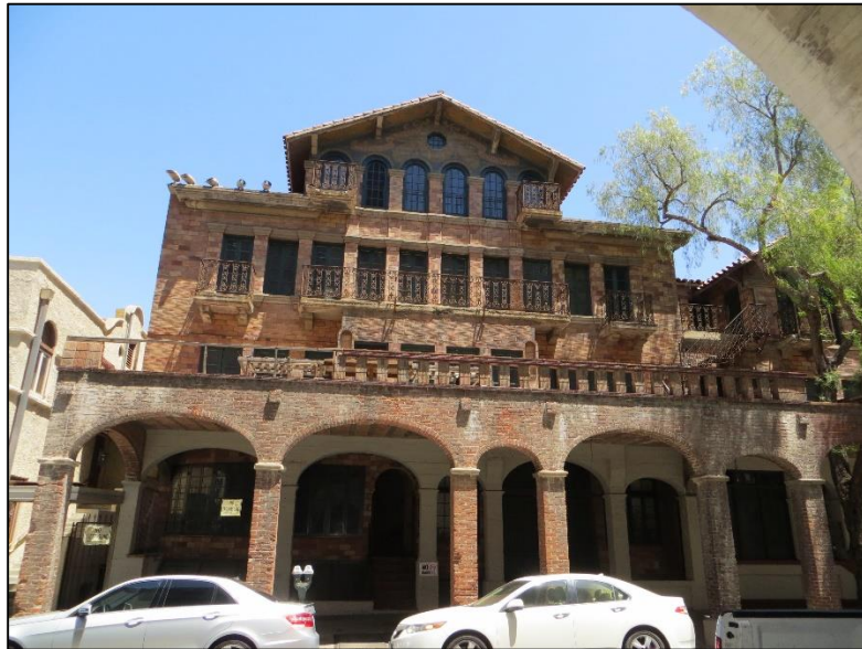
Figure 103: The Mission Inn Annex today. The left side of the balcony is crumbling and the entire exterior is plastered with “No Trespassing” signs. Photo by author.
