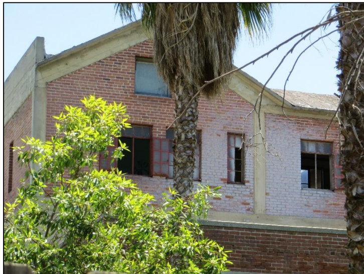
Figure 104: A side view of the Annex with broken windows, visible interior graffiti, and missing roof tiles. Photo by author.
