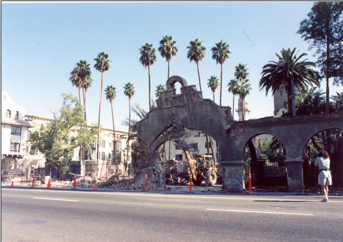
Figure 93: The hotel's front arcade along Seventh Street had to be torn down and rebuilt because it was structurally unsound. Photo courtesy Mission Inn Foundation & Museum.
