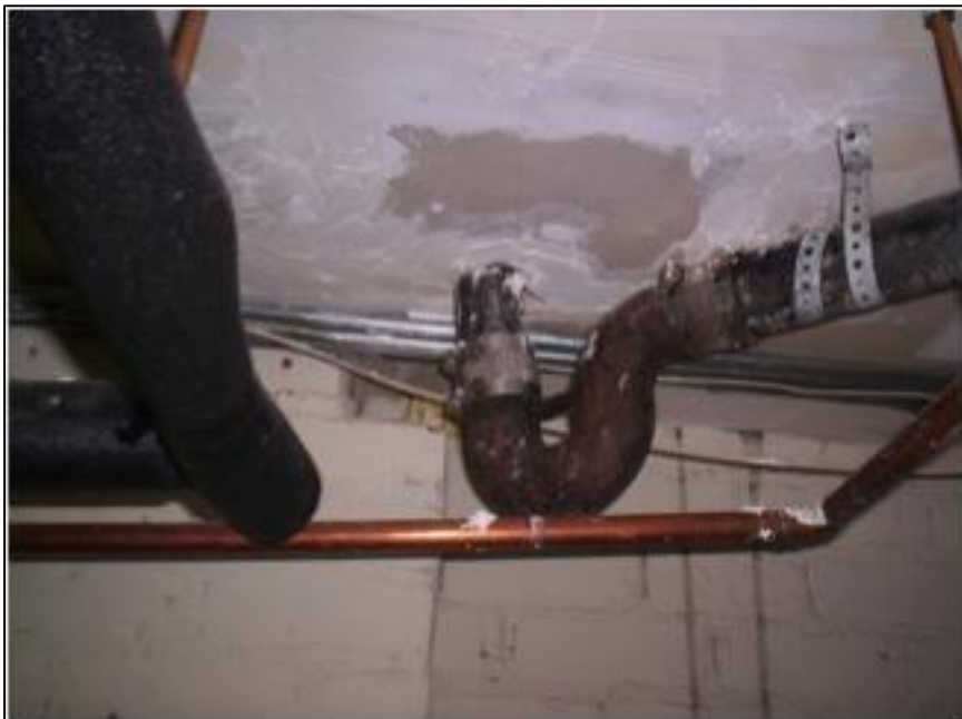
Figure 102: The overhead pipes that caused the water damage. Photo courtesy Mission Inn Foundation & Museum.
