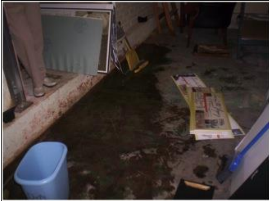
Figure 101: A water leak in 2009 made one basement storage room almost completely unusable. Photo courtesy Mission Inn Foundation & Museum.
