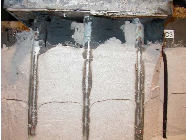
Figure 5. Side view of a pile cap after the adjacent soil has been excavated (Note the passive bulge on the uphill [right] side).
