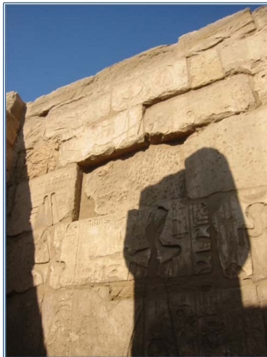
Figure 3. Peristyle court, north wall: detail of the masonry and of a “stone plate” that has fallen out.
