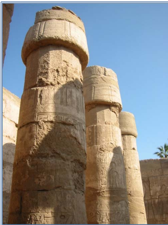
Figure 6. Peristyle court: columns with reused polygonal drums and thick layers of coating.
