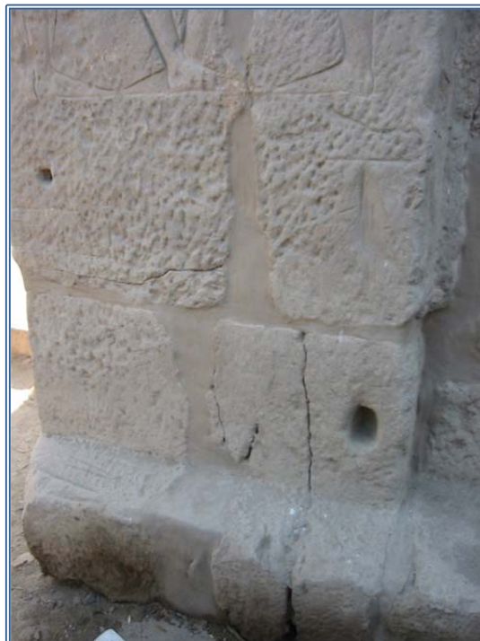
Figure 4. North door of the temple, west jamb, stone extrusion of the masonry.
