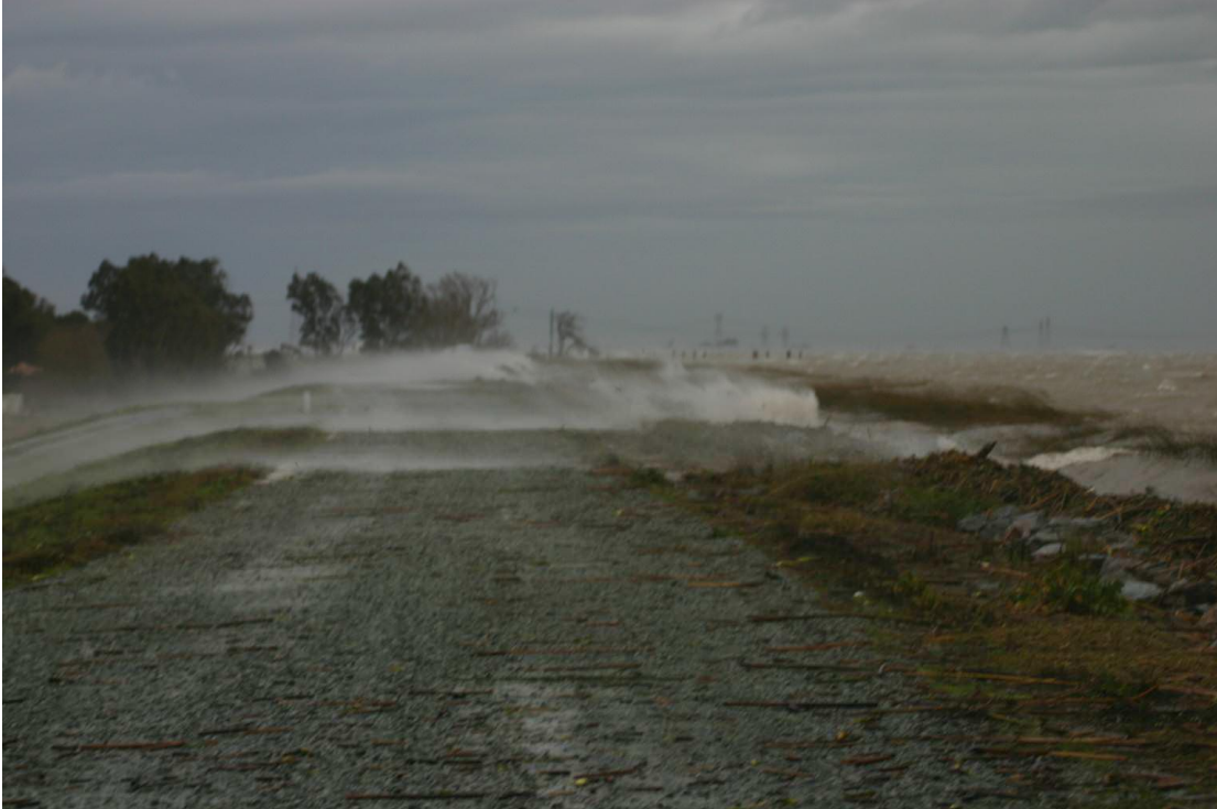
Figure P.3 Overtopping of levee, taken on Jan. 1, 2006 on Sherman Island levee adjacent to the San Joaquin River during high winds and High tide.
