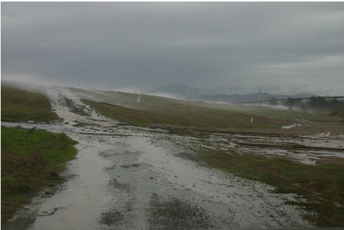
Figure P.5: Overtopping of levee, taken on Jan. 1, 2006 on Sherman Island levee adjacent to the San Joaquin River during high winds and High tide (land side)
