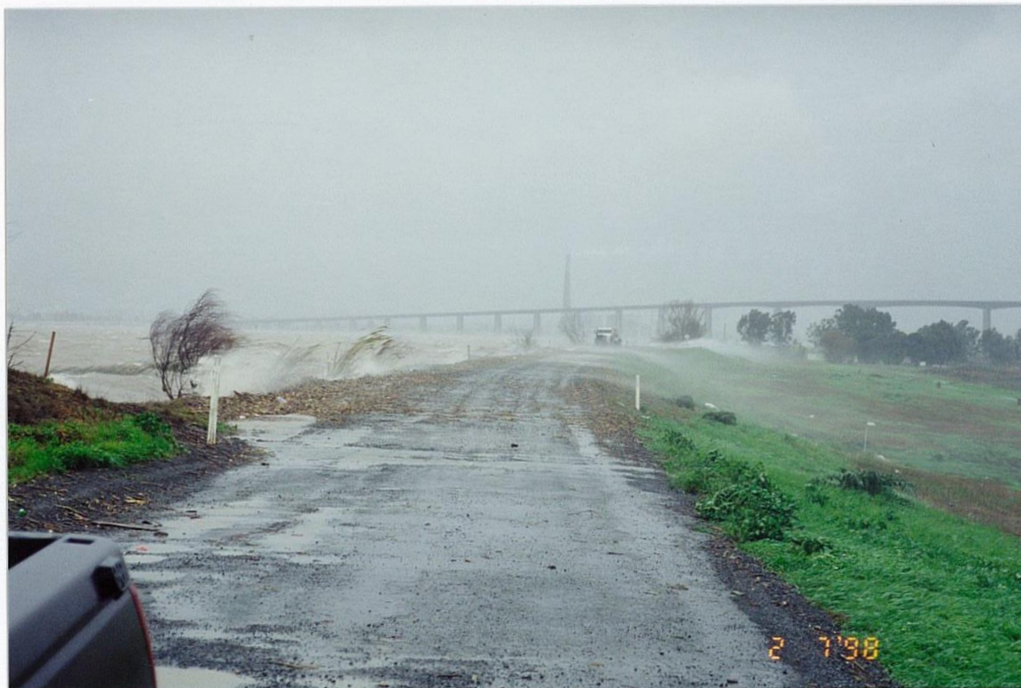
Figure P.6: Overtopping of levee, taken on Feb. 7, 1998 on Sherman Island levee adjacent to the San Joaquin River during high winds and High tide
