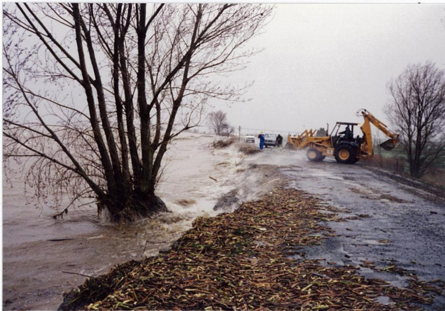
Figure P.8: Overtopping and Water side erosion of levee, taken on Feb. 7, 1998 on Sherman Island levee adjacent to the San Joaquin River during high winds and High tide
