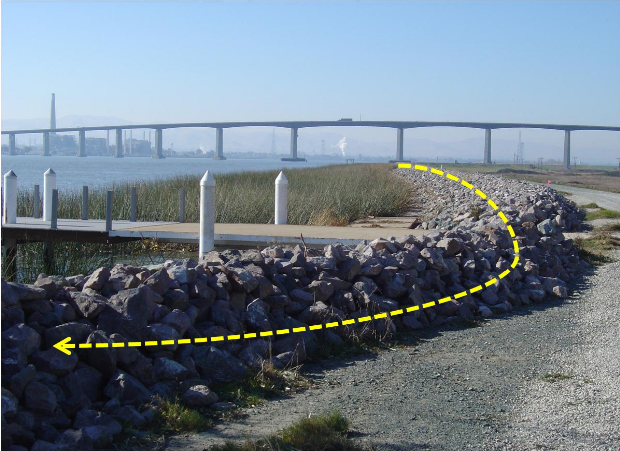
Figure 5-20: Southern Part of Sherman Island Levee System Protected with Rip-rap Armor along the San Joaquin River
