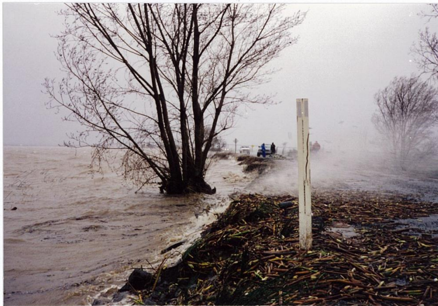
Figure P.7: Overtopping and Water side erosion of levee, taken on Feb. 7, 1998 on Sherman Island levee adjacent to the San Joaquin River during high winds and High tide.
