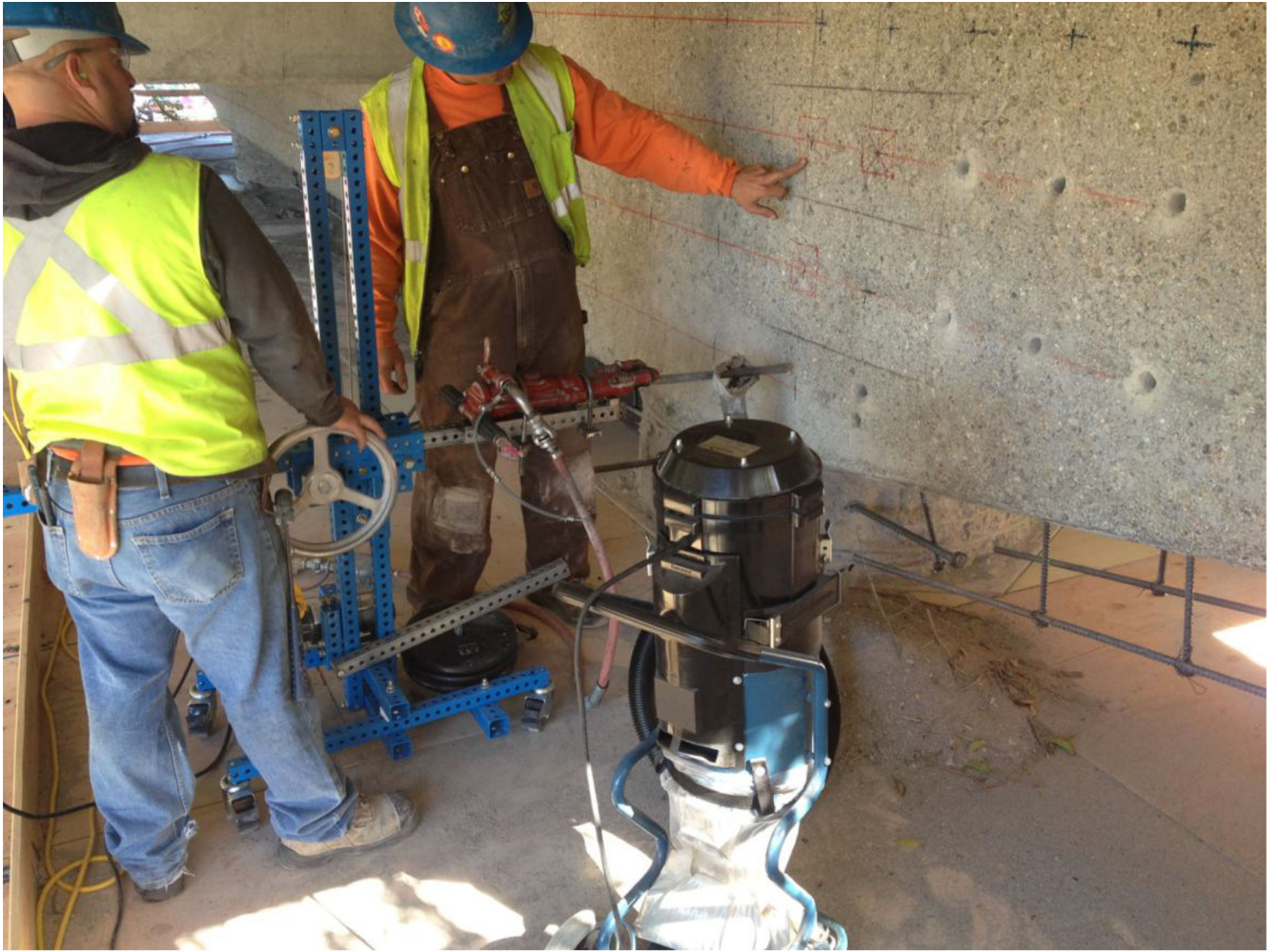
FIGURE 1. Usual method for drilling with a 36 lb pneumatic rock drill to drill hundreds of holes for structural upgrade to concrete columns supporting train tracks.
