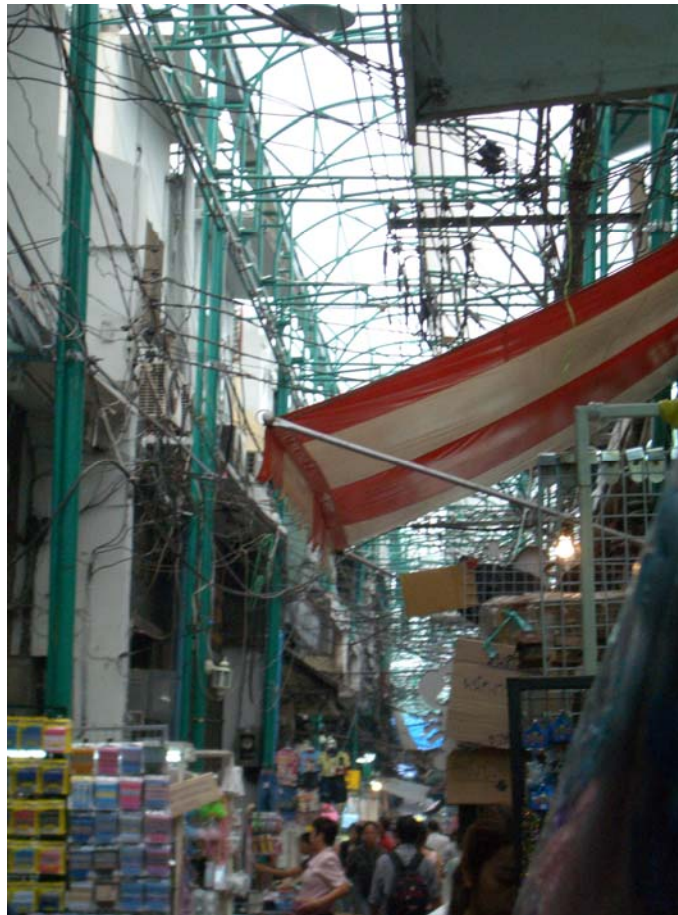
[alternative infrastructures: electrical wires in Bangkok]
