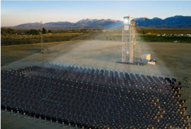
Figure 2.5: An eSolar solar thermal system in Burbank, California.
