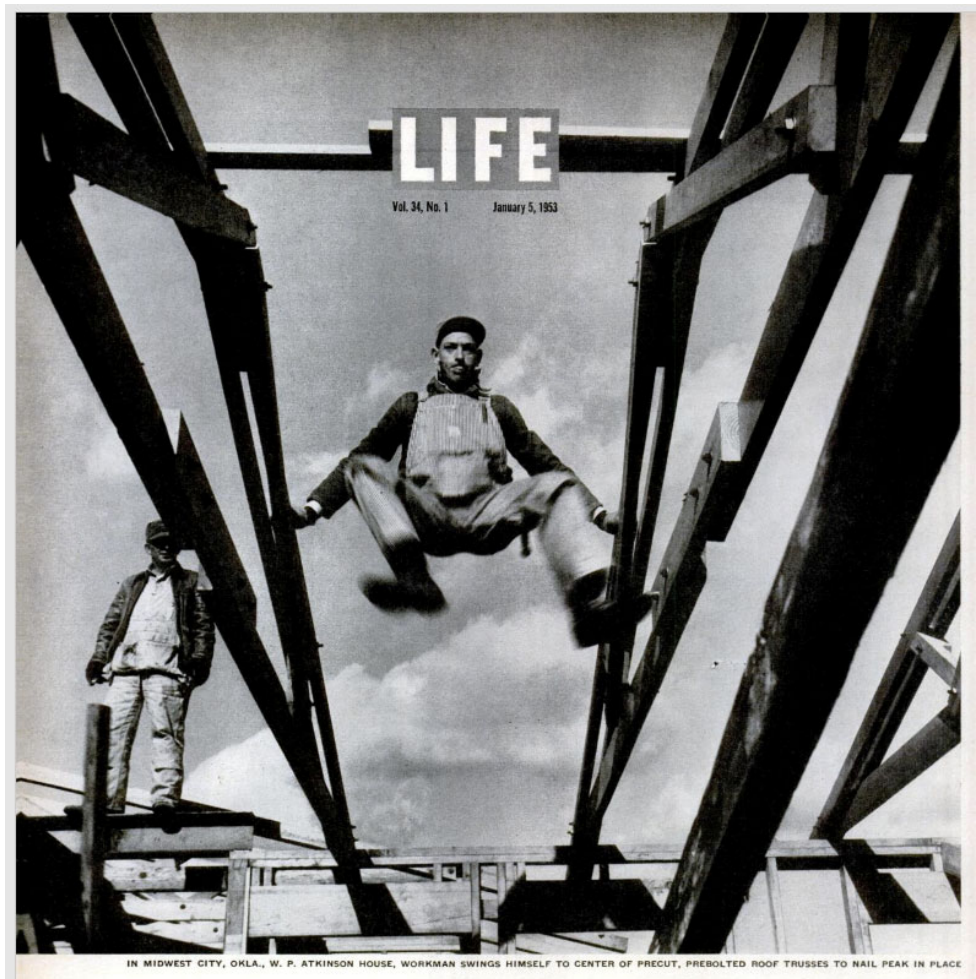
Figure 6.18. Worker swinging on nailed roof trusses on W.P. Atkinson’s Midwest City, Oklahoma Trade Secrets demonstration model. Source: LIFE , January 5, 1953, page 8.
