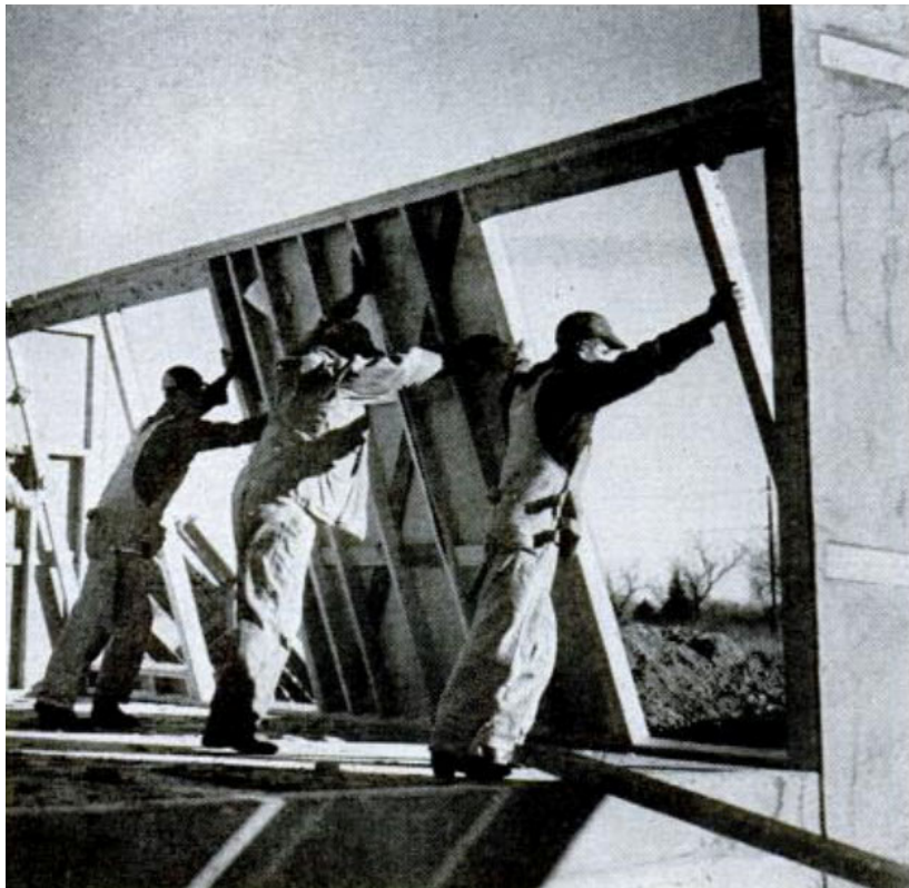
Figure 6.20. Workmen tilting a preassembled wall into place in Franklin Burns' Denver, Colorado Trade Secrets House model. Source: LIFE, January 5, 1953, page 14.
