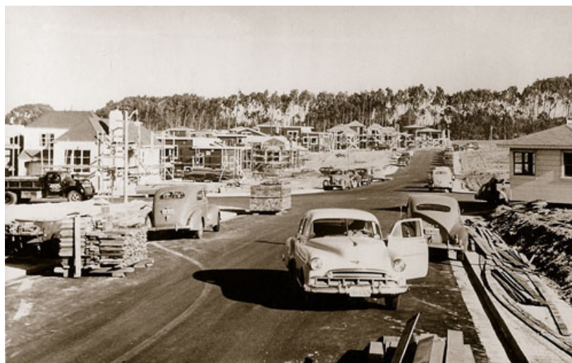
Figure 3.38. Early unit of Westlake under construction, showing house kits on curbs and houses in various stages of completion. Source: Daly City History Guild, Daly City, California.
