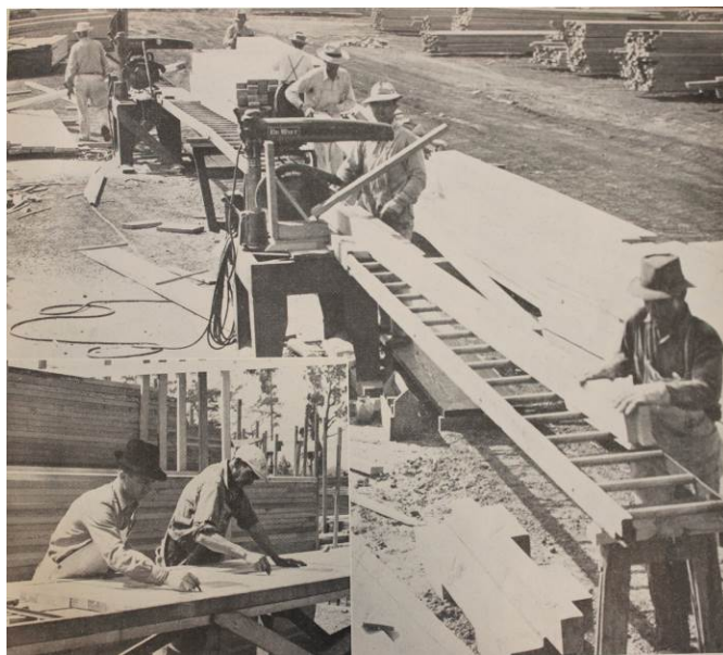
Figure 4.35. Rolling tables for precutting and keying framing and sheathing for houses at San Lorenzo Village. Source: American Builder , February 1945.
