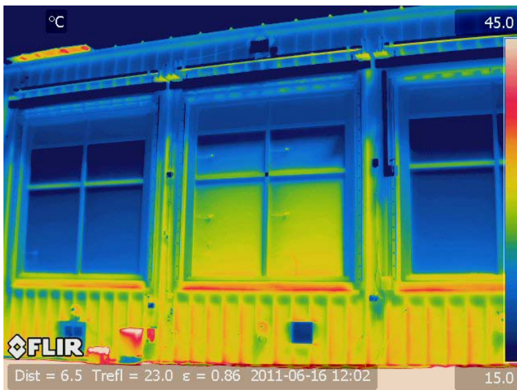
Fig. 9. Above: Outdoor view of the south-facing thermochromic window (middle room with the dark windows). Below: Corresponding infrared image showing the surface temperature of the windows (°C) on June 16, 12:02 PM ST.
