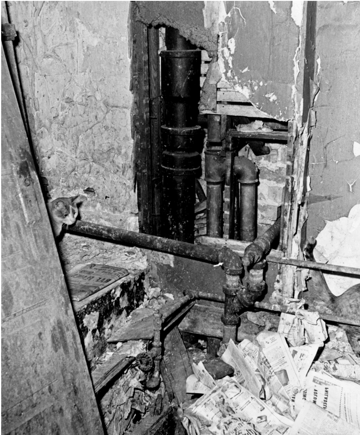
FIGURE 2.3 White Eagle Hotel, 18th and Indiana. Exposed plumbing and general deterioration! Convenient for the plumbers? Mildred Mead, April 8, 1954. University of Chicago Special Collections, apf2-09088.
