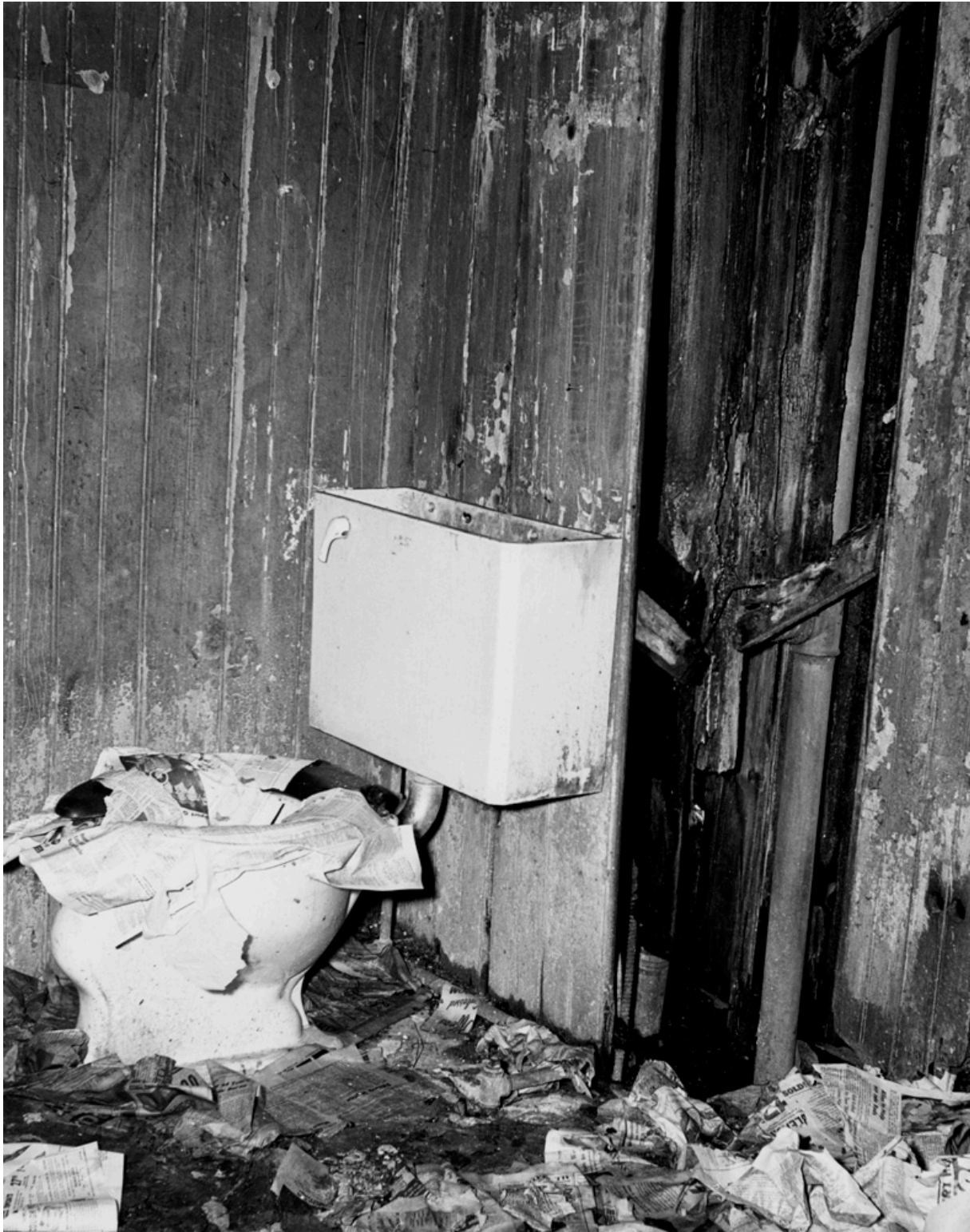
FIGURE 2.5 White Eagle Hotel converted, 18th and Indiana. This sort of condition repeated all over this building. Mildred Mead, April 8, 1954. University of Chicago Special Collections, apf2-09085.
