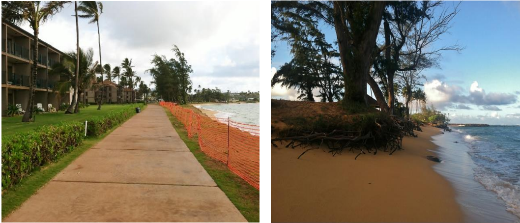
Figure 7 Kapa'a showing conditions during Summer 2012 and Summer 2014, respectively. Note the proximity of infrastructure to the beach and the existence of a temporary fence to slow erosion of the coast along this section.
