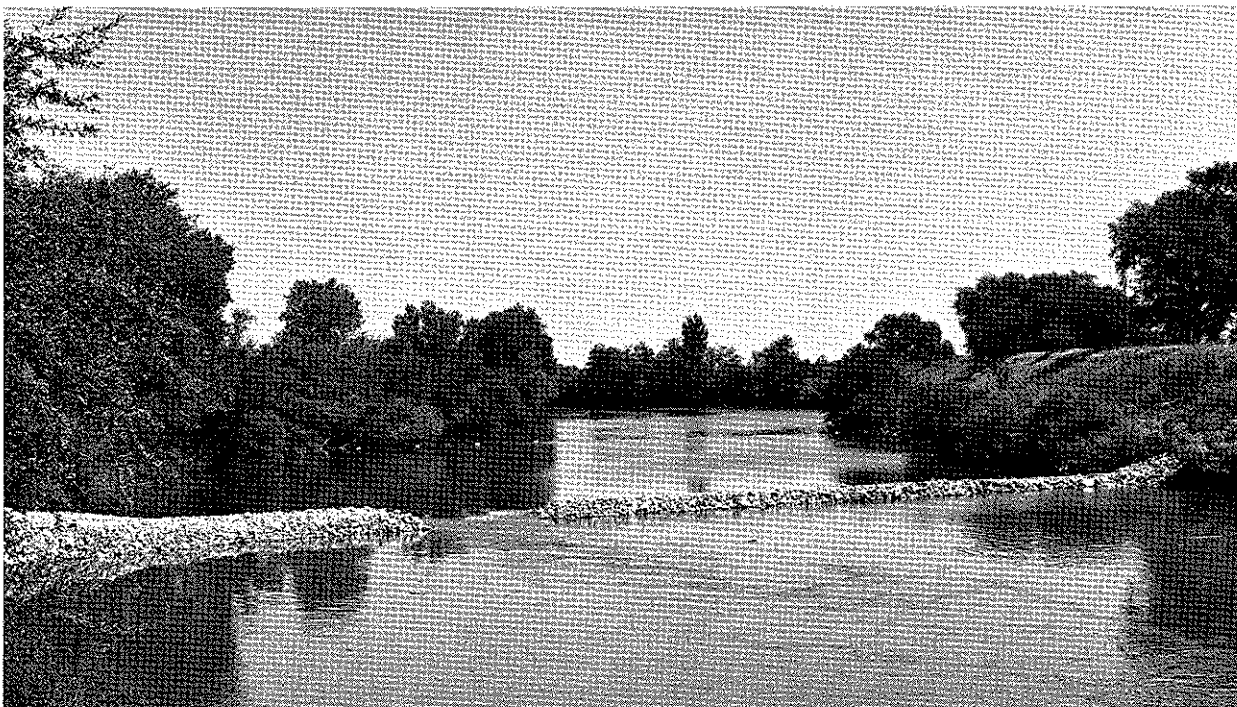
Sutter Slough rock barrier. In late summer, 1976, the Department of Water Resources installed an emergency rock barrier in Sutter Slough to force more of the Sacramento River's flow past the Delta cross-channel at Walnut Grove, where water could be diverted to the San Joaquin Delta.
