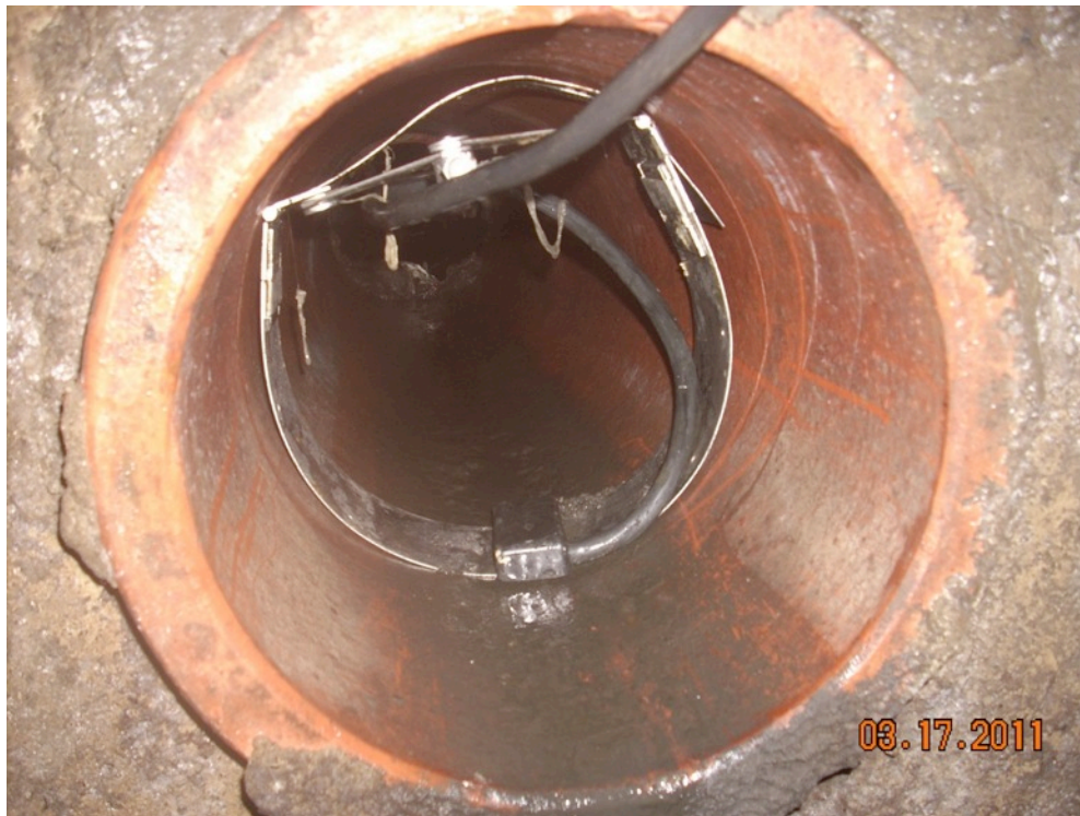
Figure 12. Flowmeter installed in lateral pipe at Cesar Chavez and Harrison
