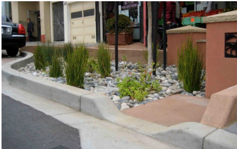
Figure 6. Bioretention planter with stormwater inlet
