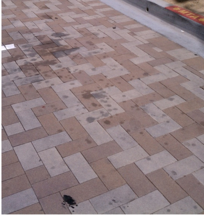
Figure 13. Oil stains on permeable pavement parking strip
