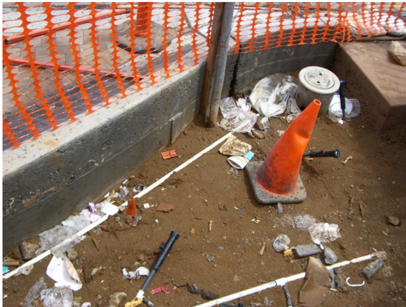
Figure 11. Trash thrown on permeable pavement subgrade
