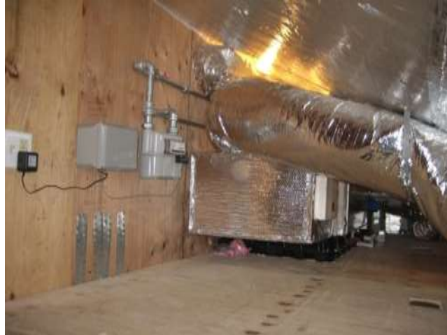
Image 33 - P7 New Furnace and Ductwork in Sealed Attic
