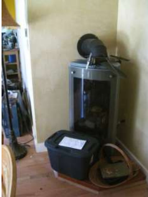
Image 25 - P6 North, Gas Point Source Heater, Direct Vent, Sealed Combustion
