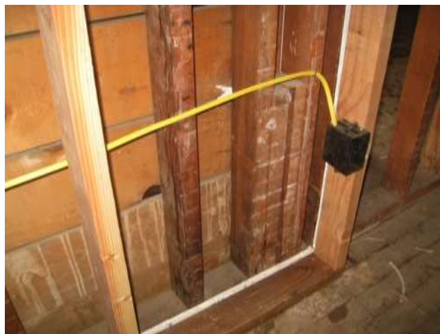
Image 20 - P6 Double Stud Wall Framing with New Wall Built to Inside of Existing
