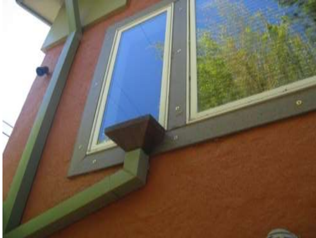
Image 13 - P4 Simple Grey Water Collection System at Kitchen Window
