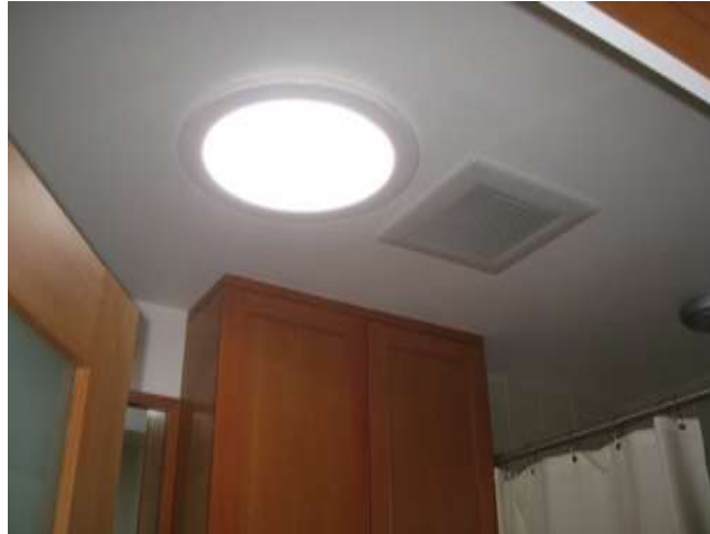
Image 46 - P10 Solar Tube for Daylighting in Bathroom
