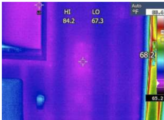
Figure 7 - P1 thermal bridge at deck support bracket
