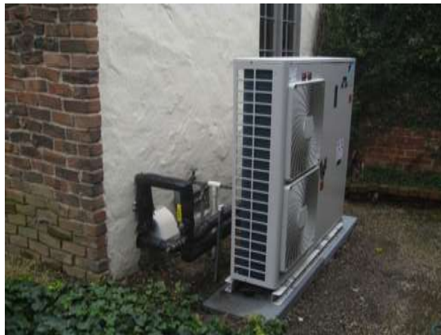
Image 7 - P2 Replacement Heat Pump Outdoor Unit
