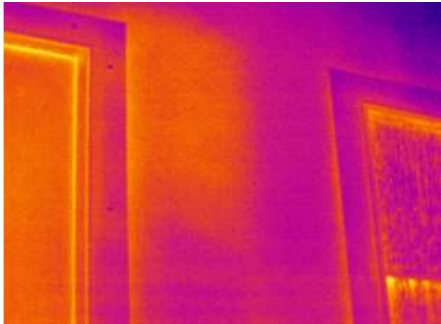
Figure 62 - P4 missed insulation around bathroom window
