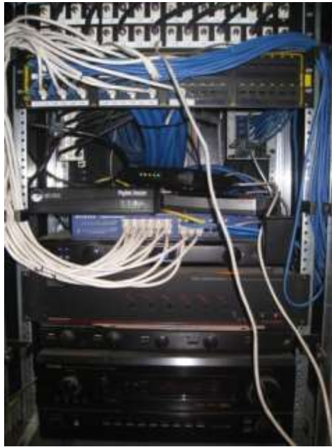
Image 8 - P2 AV and Data Equipment in Basement Cabinet
