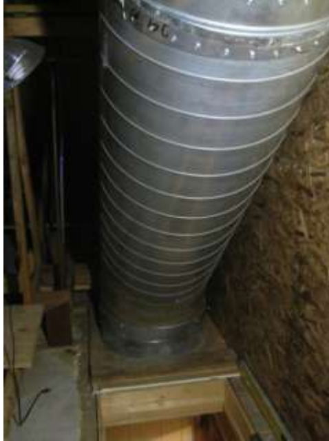
Image 11 - P4 View of Large Natural Stack Vent Duct at Top of Stairwell
