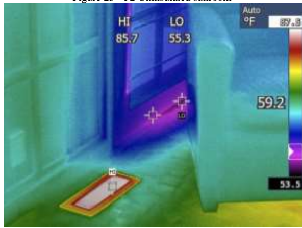
Figure 26 - P2 sunroom radiant floor and register next to leaky door
