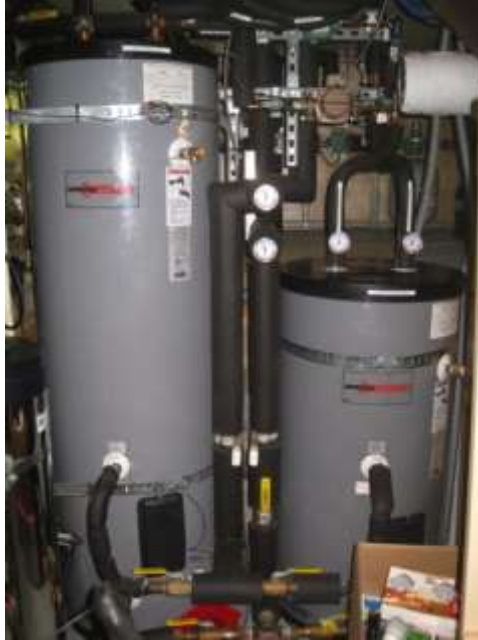
Image 6 - P2 Heated and Chilled Water Storage Tanks in Basement
