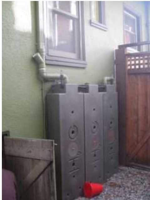
Image 35 - P8 Rainwater Collection Storage
