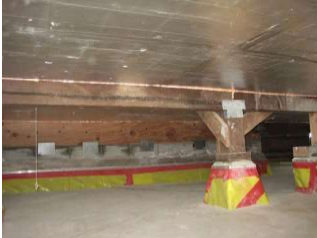
Image 30 - P7 Crawlspace with New Slab, Foam Board Insulation, Structural Reinforcement, Air Sealing and Water Proofing
