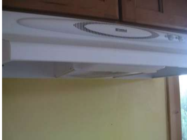
Image 16 - P5 Kitchen Range Hood Exhaust
