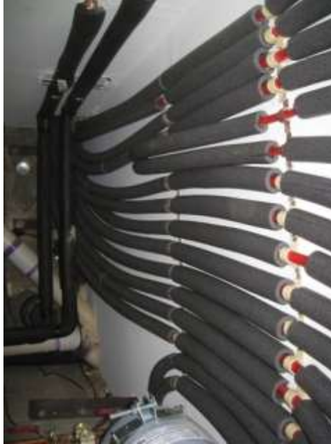
Image 45 - P10 Space Heating Distribution Pipes, Insulated but with Large Gaps, in Garage
