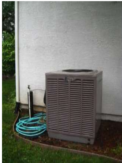
Image 40 - P9 Outdoor Evaporatively Cooled Condensor
