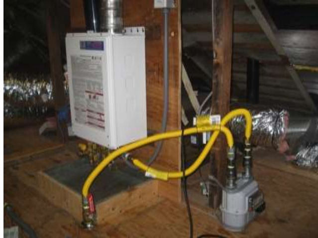
Image 2 - P1 Tankless Gas Water Heater in Attic with Gas Submeter
