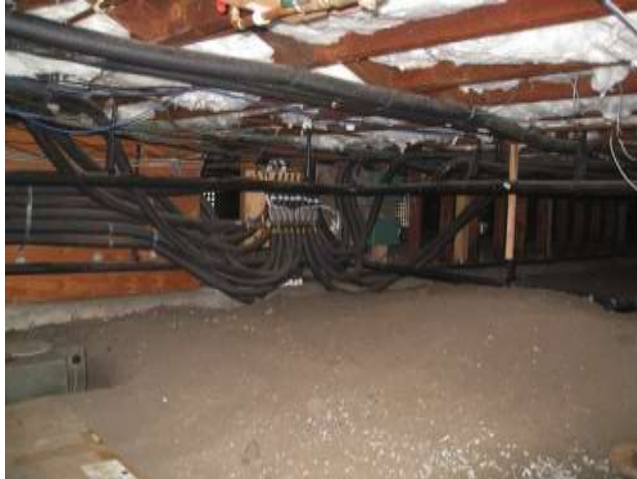
Image 38 - P8 Crawlspace, with Fiberglass Batts in Ceiling and Insulated Hot Water Distribution System
