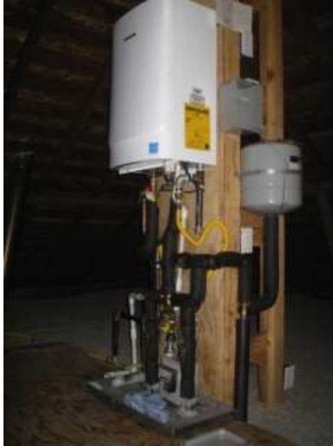
Image 27 - P6 South, Gas Tankless Water Heater with Solar Thermal Pre-Heat
