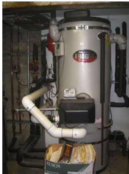
Image 44 - P10 Solar Combisystem Tank in Garage
