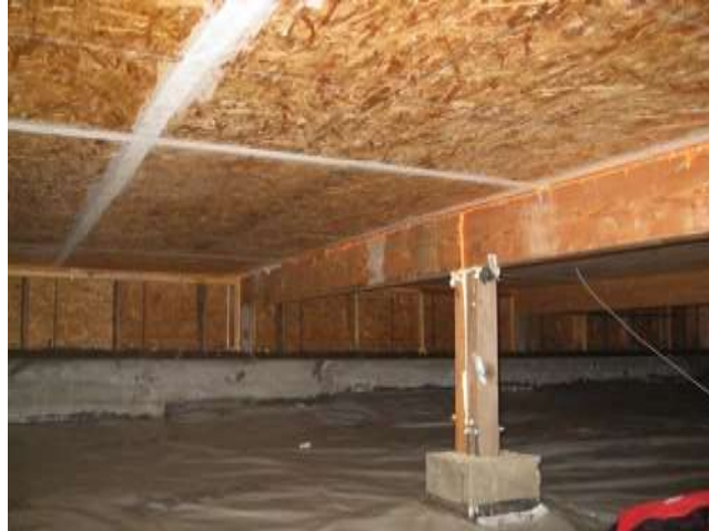
Image 15 - P5 Sealed Crawlspace
