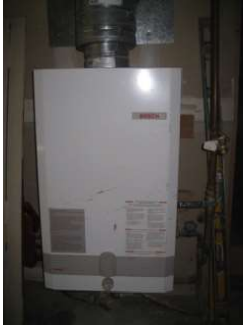
Image 12 - P4 Tankless Gas Water Heater in Garage, Atmospherically Drafted
