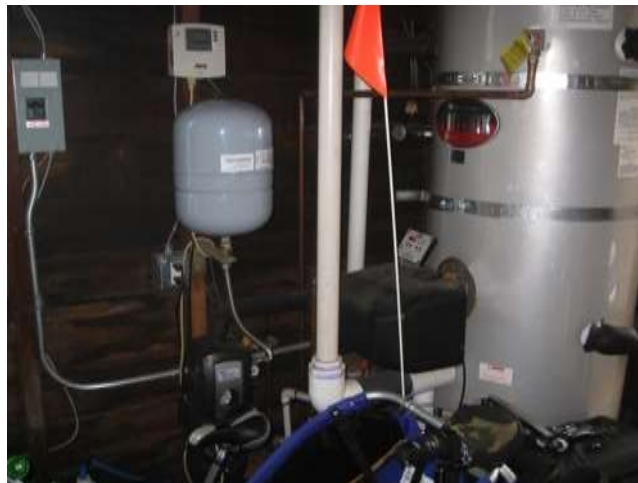
Image 37- P8 Solar Combisystem Storage Tank in Garage
