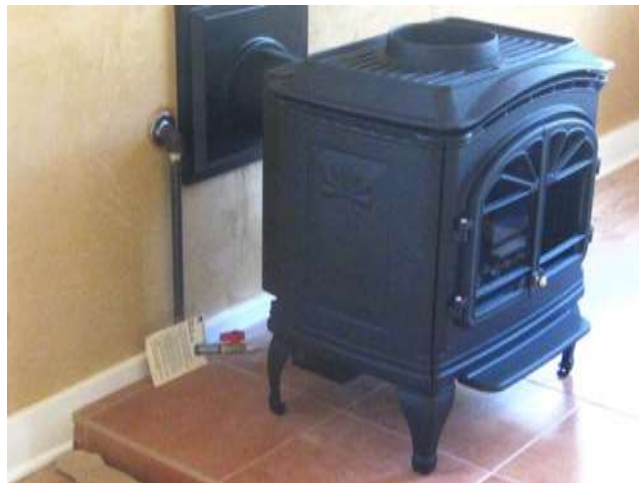
Image 26 - P6 South, Gas Point Source Heater, Direct Vent, Sealed Combustion
