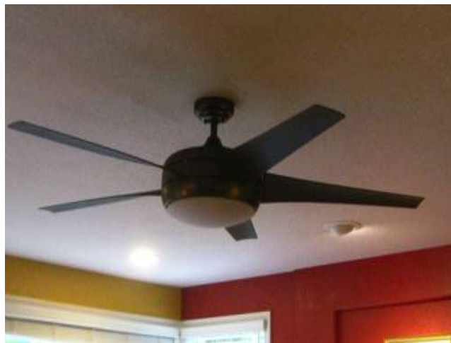
Image 42 - P9 True Airfoil Ceiling Fans to Assist In Non-Compressor Cooling
