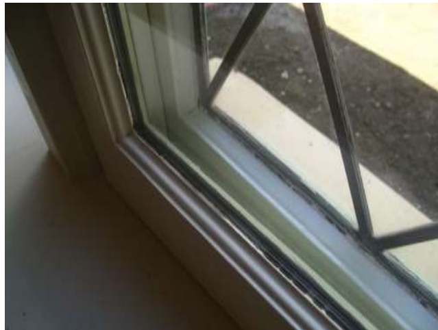
Image 22 - P6 South, Existing Wood Frame Windows Rehabbed with Second Pane of Glass
