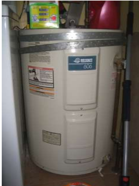
Image 18 - P5 Electric Resistance Water Heater in Laundry Room
