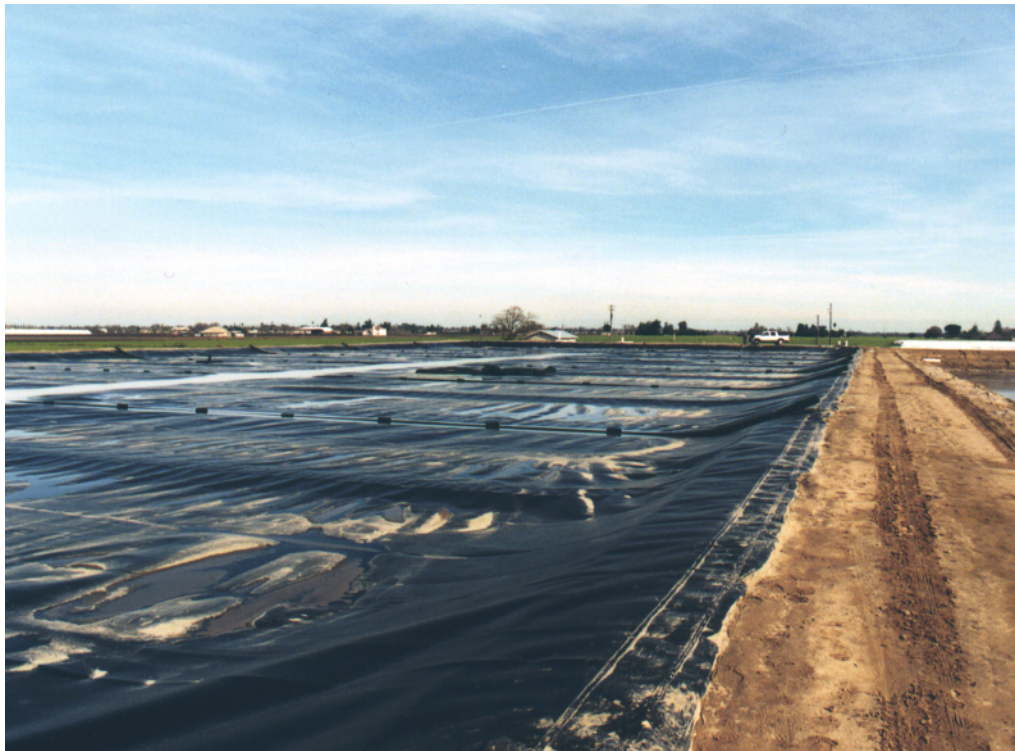
Figure B-2 Photograph of Castelanelli Bros. Dairy covered lagoon digester located in Lodi, CA. (source: RCM Digesters, Inc.)
