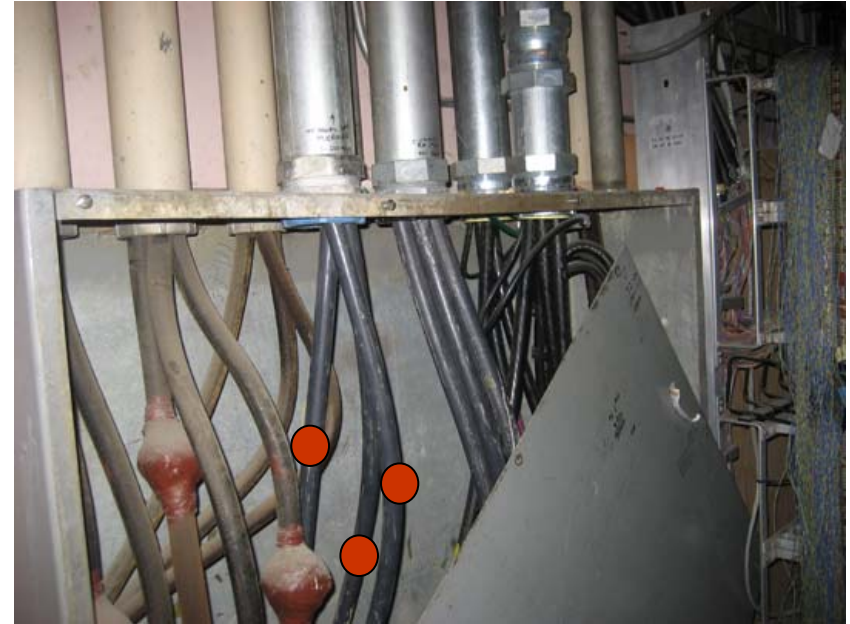
Current sensors on slack 480-volt 3-phase cables in Cory Hall
