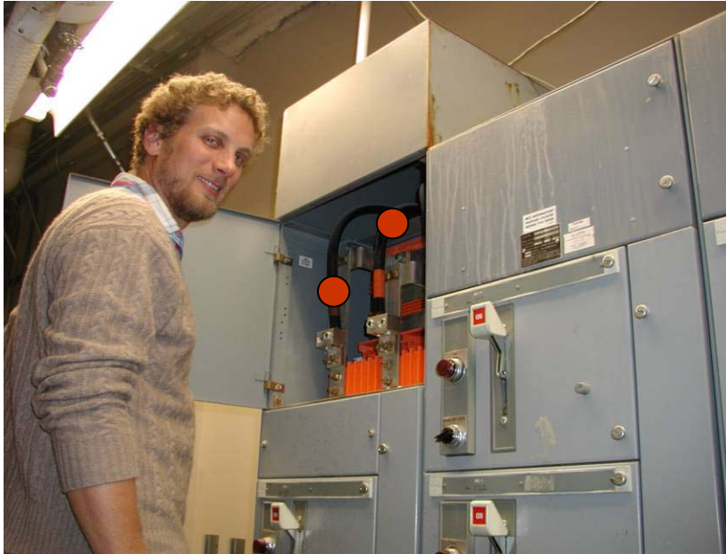
480-volt 3-phase cables that supply the Berkeley Microfabrication Facility in Cory Hall
