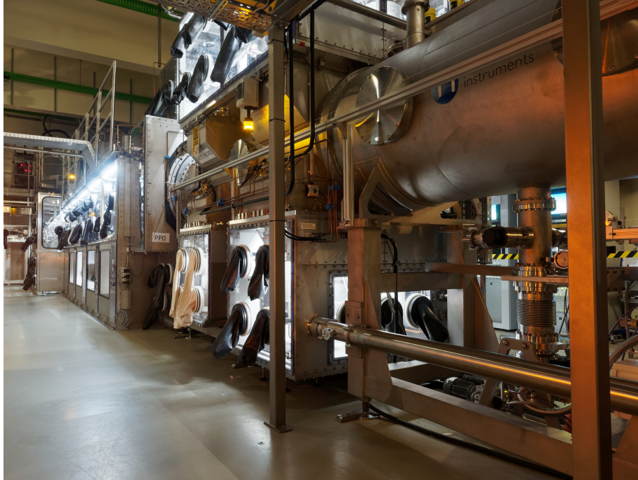
Figure 13: A View along the beam line. Shown on the right side is a part of the WGTS magnet cryostat with the glove boxes around the DPS1-F pumps (top and bottom). To the left follows the glovebox system around DPS and CPS .
