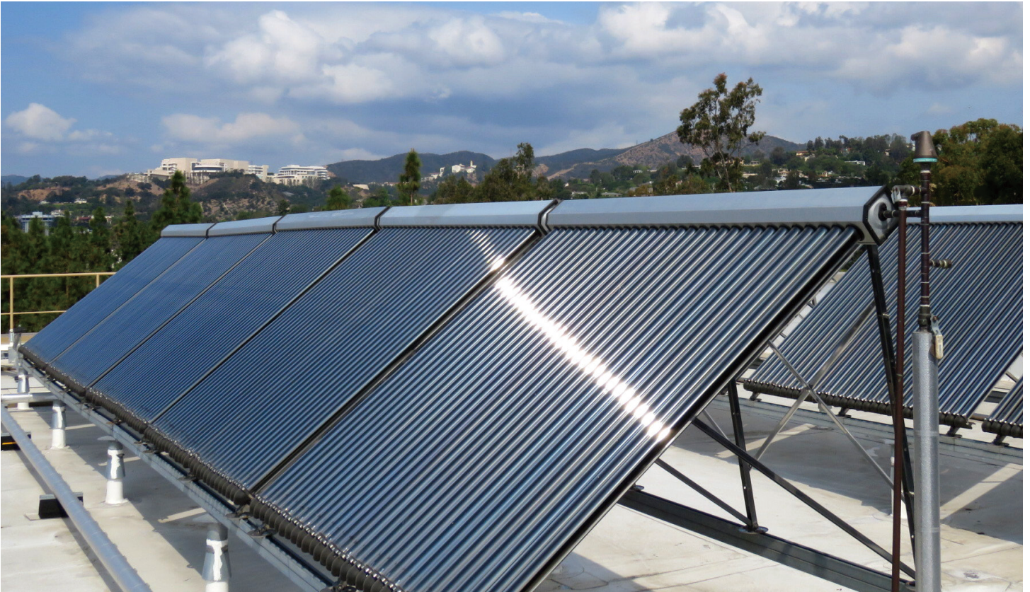
Solar Water Heating at UCLA Residence Halls (Photo credit: Nurit Katz)
