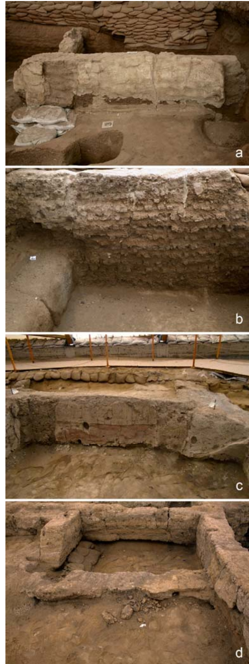
Fig. 2 Conservation issues in the North Area: (a) plaster delamination in F.230 (b) surface erosion in F.225 (c) wall undercutting in F.1617, and (d) collapse in F.2106. Source (a)-(d): Ashley Lingle. Source: HIVE Lab
